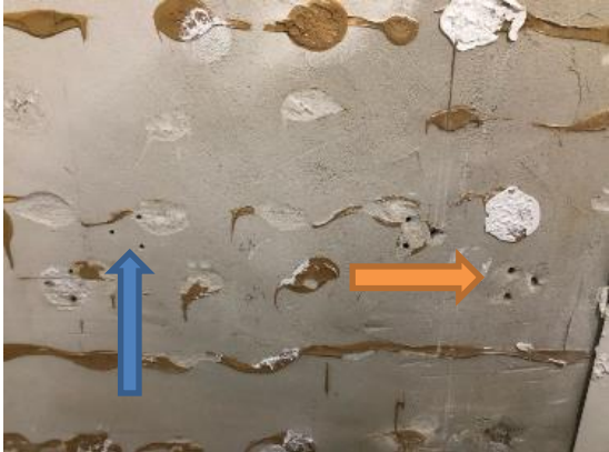
Screw holes in plaster not the metal plate
