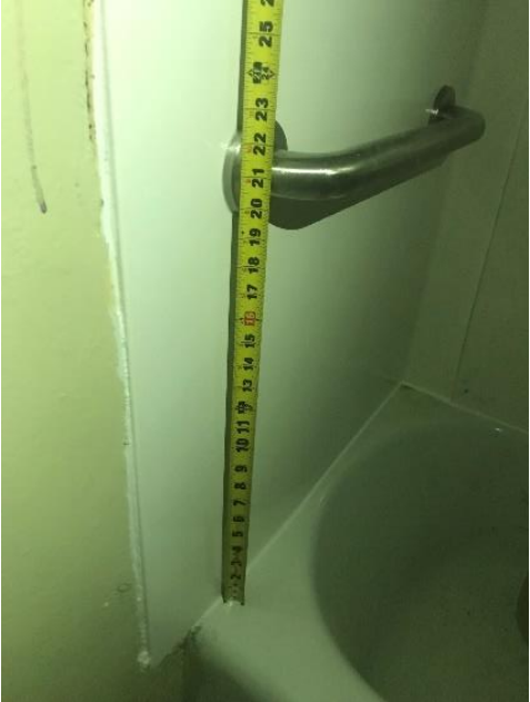
Grab Bar installed too low & not into metal anchor plate
