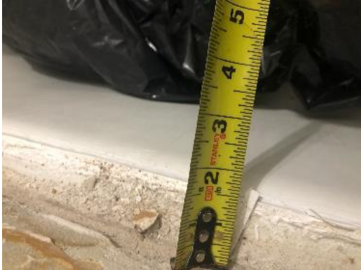
Gap between Tub and Enclosure
