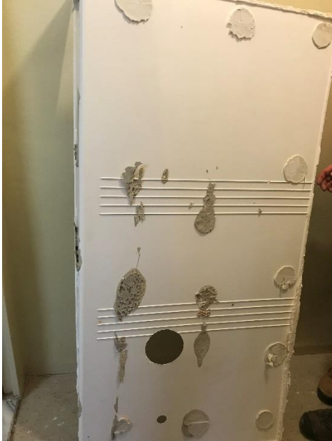
Unevenly applied adhesive
