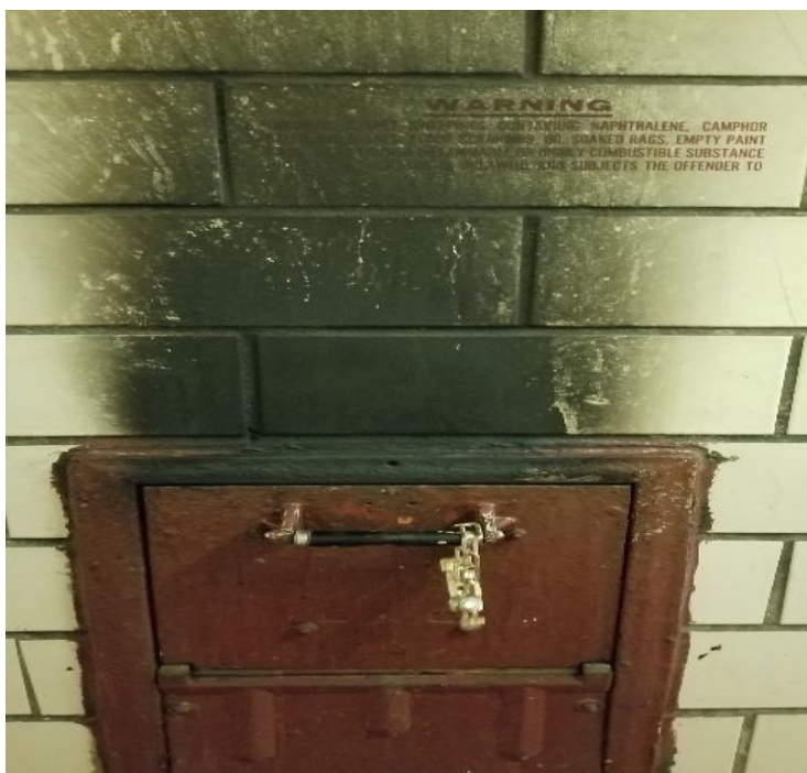
Unsecured fourth floor hopper door where the September 4 fire began
