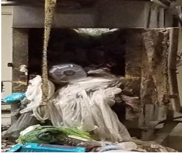
Garbage in the compactor room backed up
