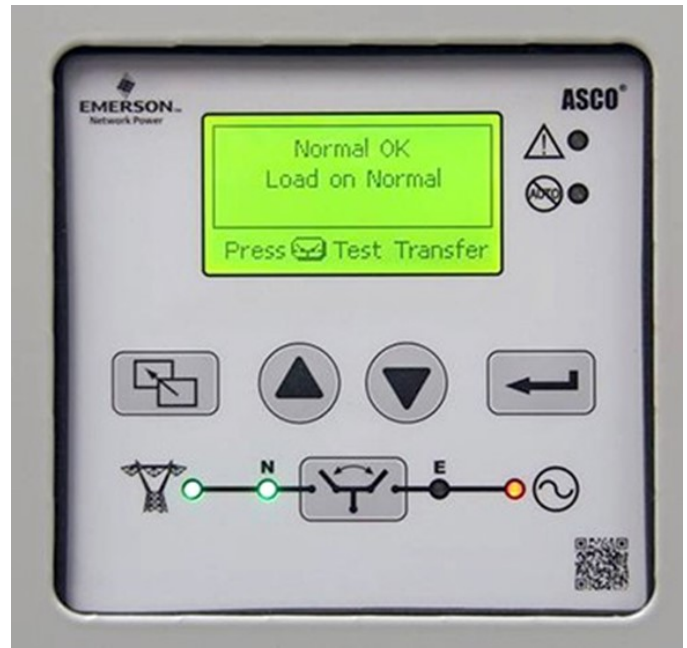
ASCO transfer switch control panel.
