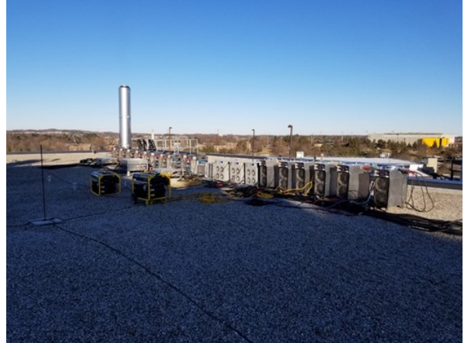
No street access required suitcase load banks brought up to the roof to test a 2.2MW 600v gen-set.
