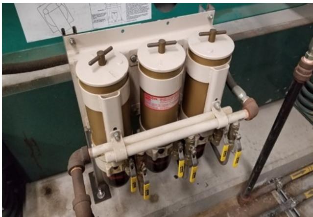
After market diesel filtration system.
