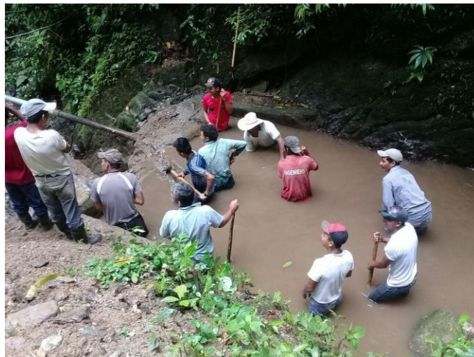
Men from the village of El Zapote working on their new water system.
