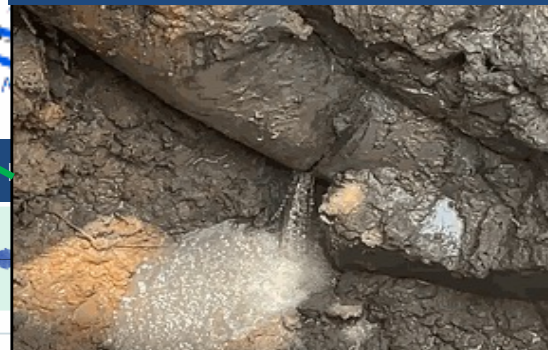
Leak on Bend (haunched)
