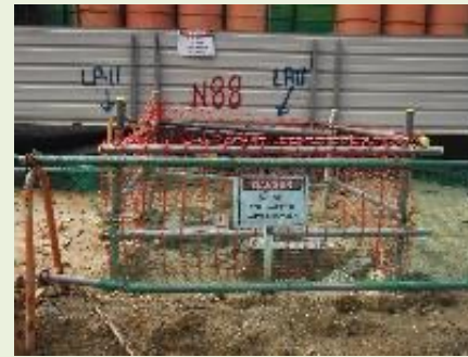
Water valve tagged and demarcated on site
