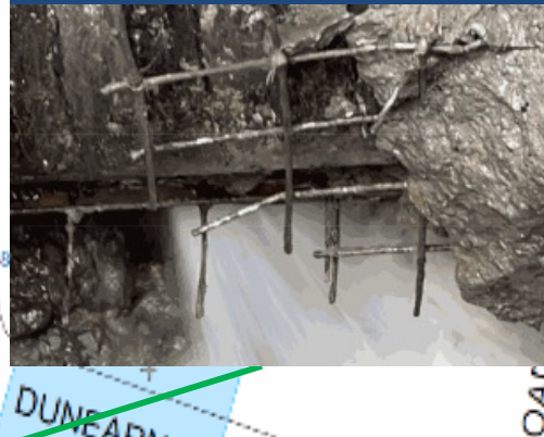
Leak on pipe body
