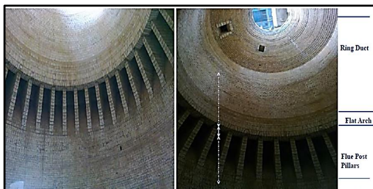
Fig.1.2: View of CDQ Pillar, Flat Arch & Ring Duct
