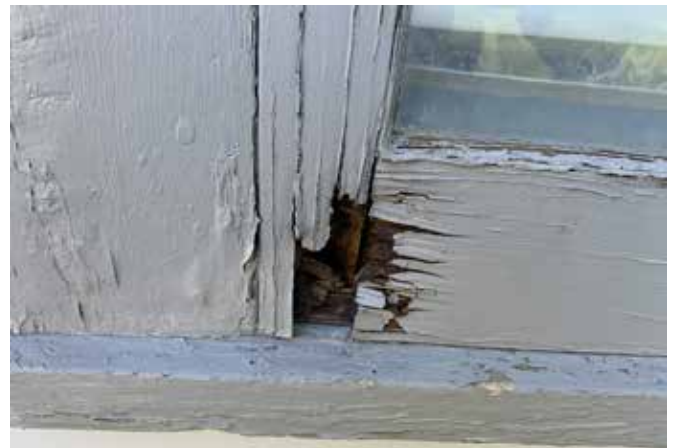
A rotted window frame on one of Pa's windows at the Ingalls Home on Third Street.
