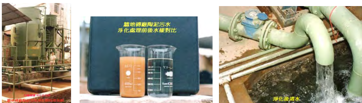
Figure 14. SPR System for wastewater reusing of ceramic manufacturing plant. (CHINA)
