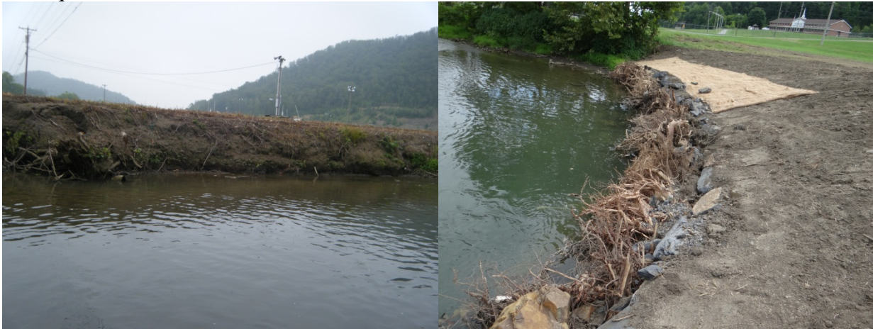
Figure 6. Before restoration (left) stream bank was eroding at a cut bank at Earhart Campground. After (right), root wads and foundation rocks support the stream bank.
