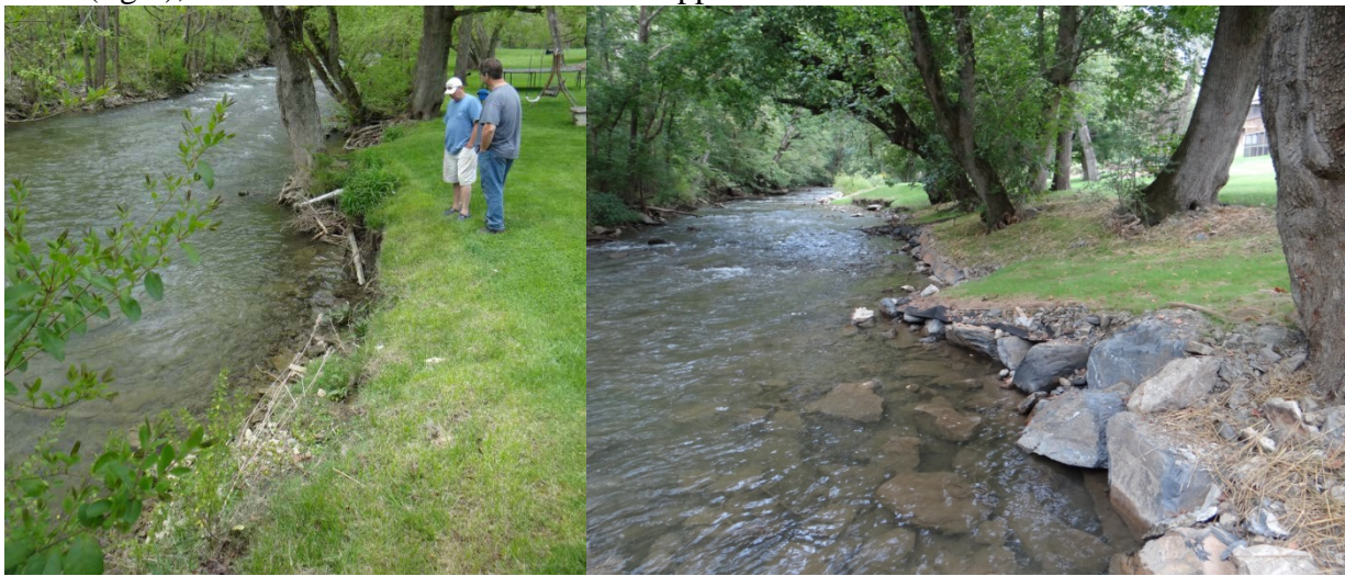
Figure 7. Before restoration (left) stream bank was eroding at this residential property. New rock vanes protect the bank and divert water back toward the center of the channel.
