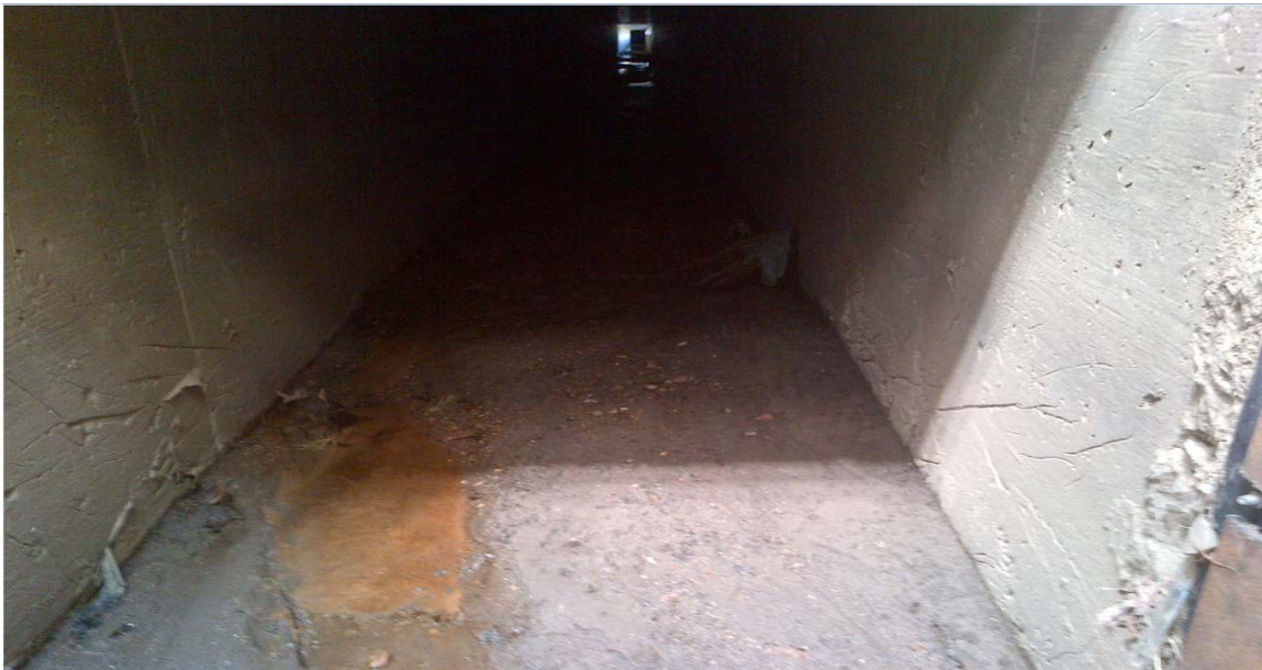
Figure 2: Sediment in 5' x 4' Box Culvert
