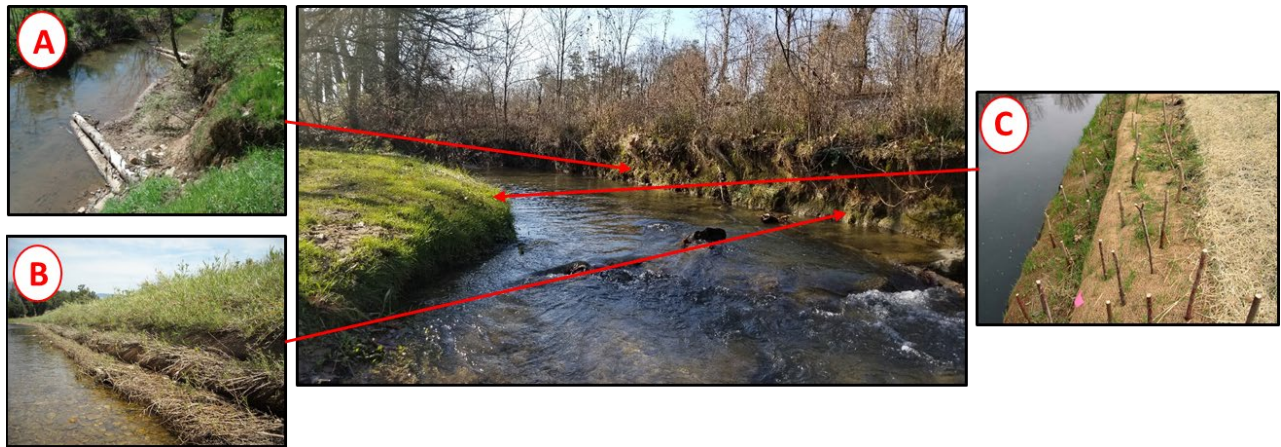
Figure 3: Site 2: vertical banks and undercutting. A: log-vane to redirect stream flow toward the center. B: bank shaping. C: bank shaping, matting and live-stake planting.
