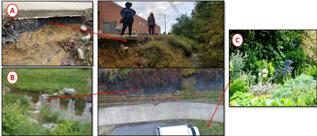
Figure 5: Site 4: undercutting. A: backfilling and bank shaping where the Millennium Trail is undercut. B: cross-vane installation. C: rain garden.
