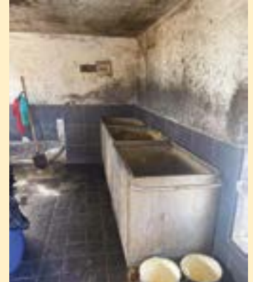
The preparation room needed a lot of work. Happy Paws have paid for a complete refurbishment of the building. This will provide a clean, safe working environment so food and medicines can be prepared.
