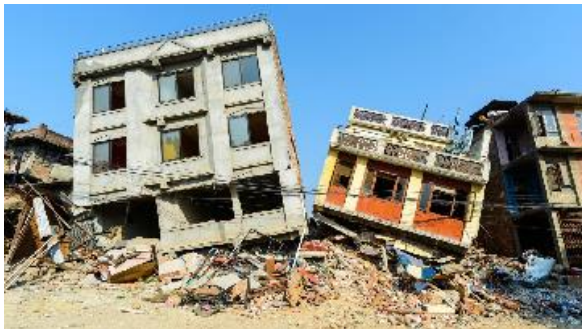
The aftermath of the Nepal earthquake in 2015. Collapsed buildings in Kathmandu. (Image credit: dutourdumonde via Getty Images)
