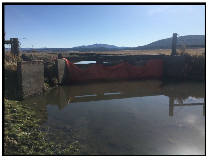
Exhibit 2: October 2019 – Irrigation Diversion looking downstream to the south. Tarp is used to support leaky drop boards. Structure will be replaced with a fish ladder constructed west side of diversion.
