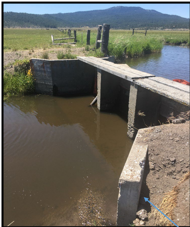
Exhibit 3: June 2020 – Irrigation Diversion looking to the northwest as drop boards are in place diverting water to the east ditch system. Erosion around structure as high spring flows overtop dam.
