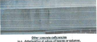
Other concrete deficiencies (e.g., deterioration at edges of beams or columns, spalling, rust spots due to holes or cracks)
