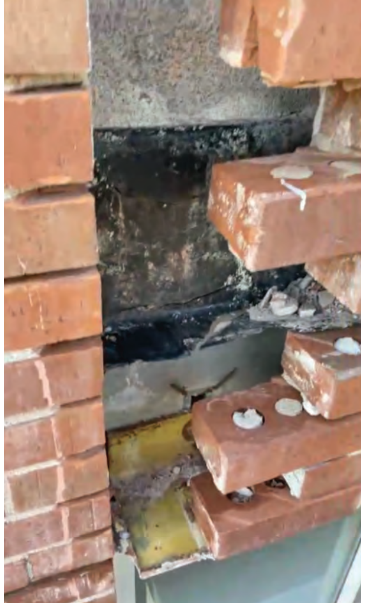
2. Opening above lintel showing existing PVC flashing.
