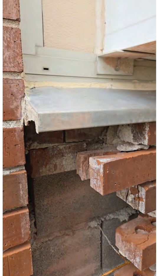
8. Window bump-out brick anchored below the extra brick layers.
