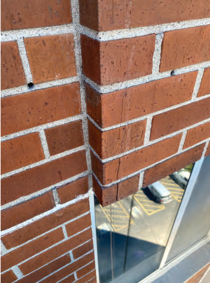
9. 11-story north wall larger crack at bump-out extends into finer cracks requiring expanded repair (typical).
