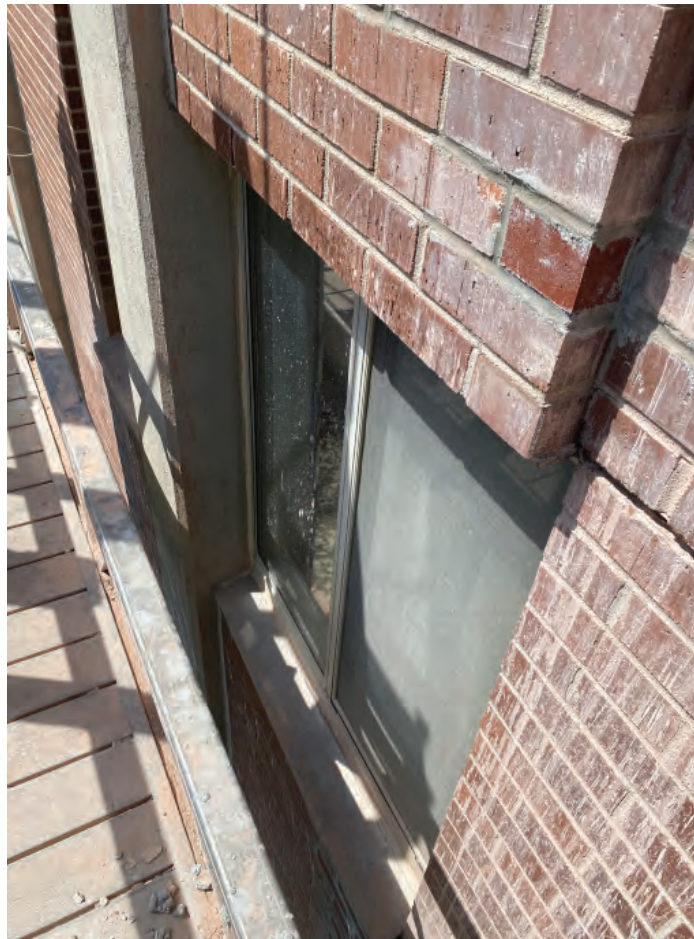
6. 11-story south wall brick water splash on window (typical).
