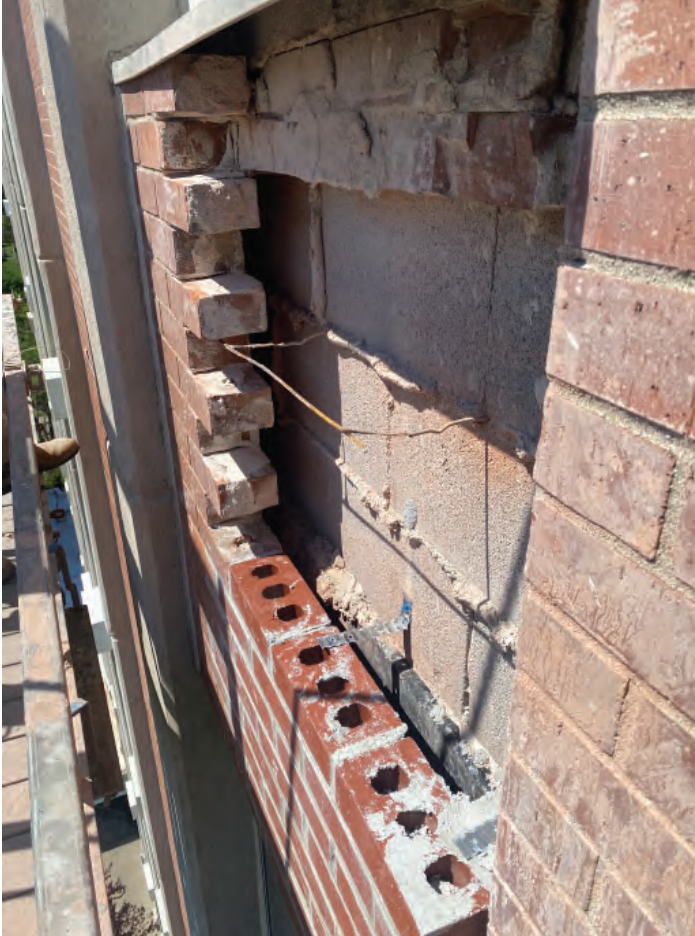
3. 11-story south wall nearly full width brick replacement right of Column 11-13 at 11th floor window bump-out.
