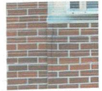
Vertical cracking in masonry above or below windows
