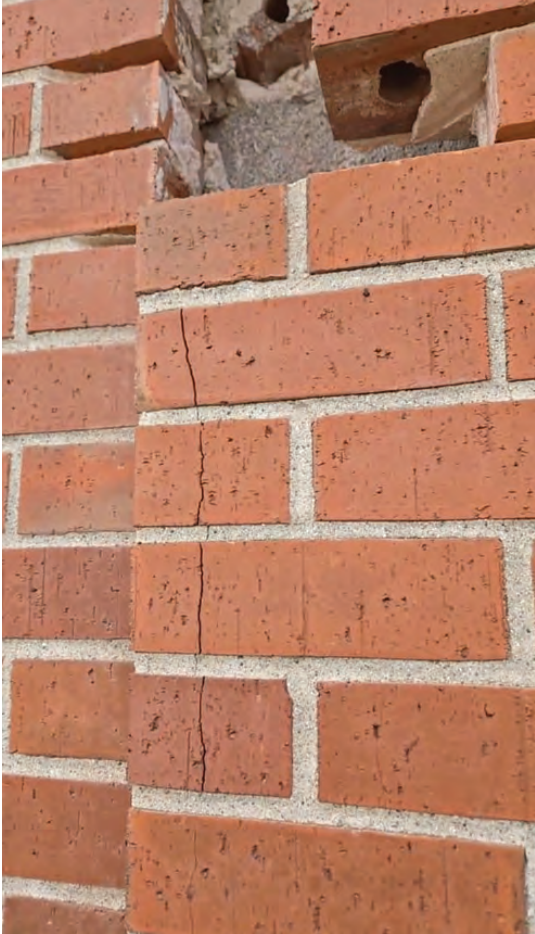
3. Additional brick cracks not in Drawings.
