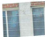
Other concrete deficiencies (e.g., deterioration at edges of beams or columns, spalling, rust spots due to holes or cracks)
