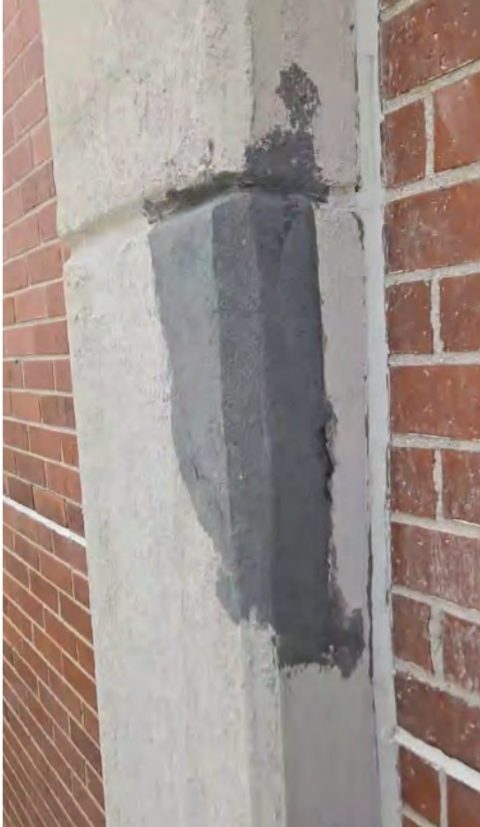
5. Column larger cracks require patching.
