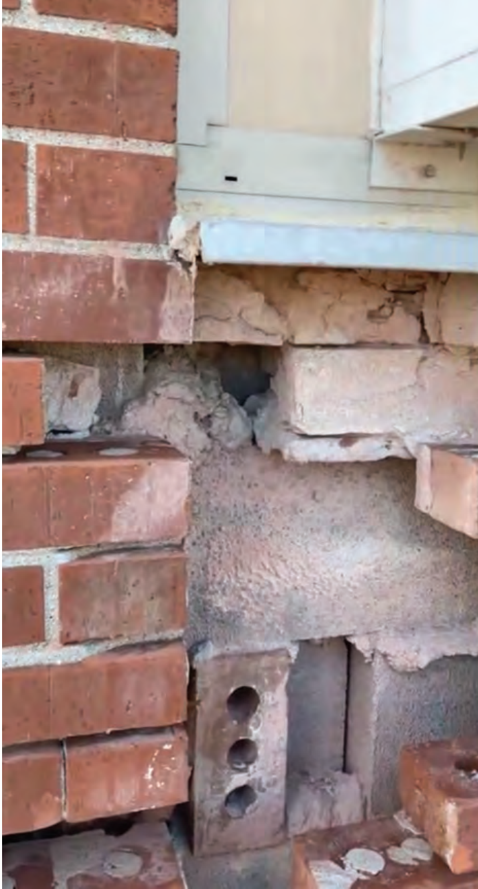
3. Opening below window showing additional brick layers.
