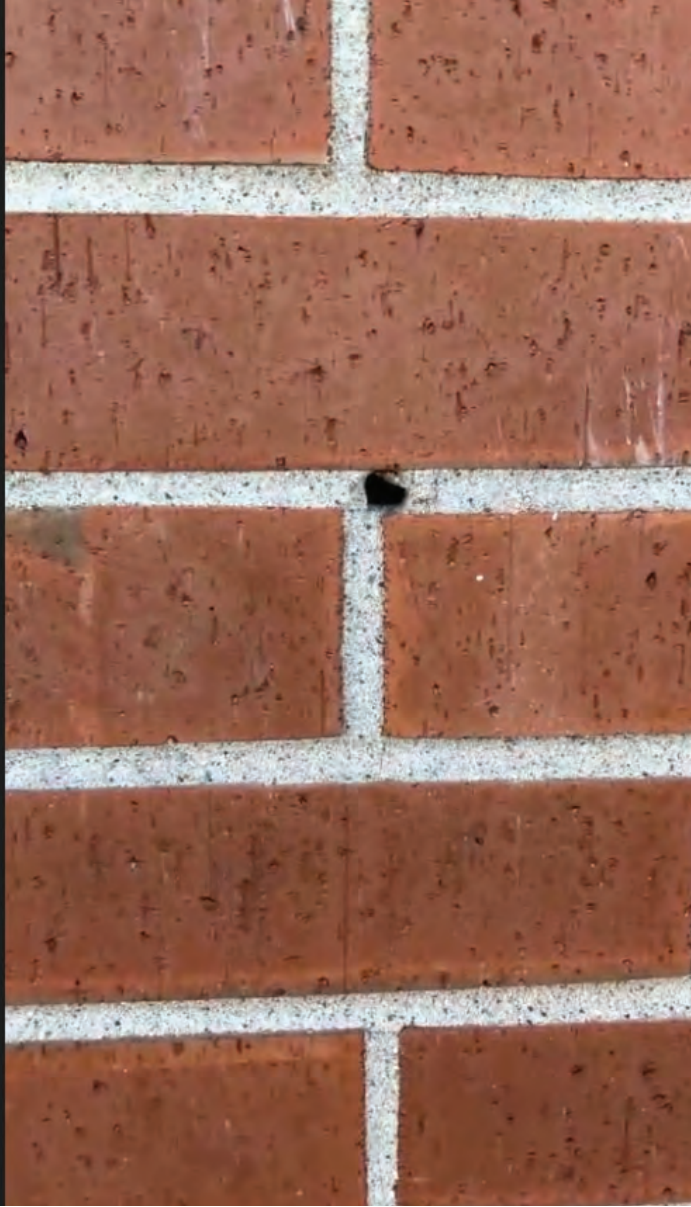
7. Weep hole without visible wick (typical).
