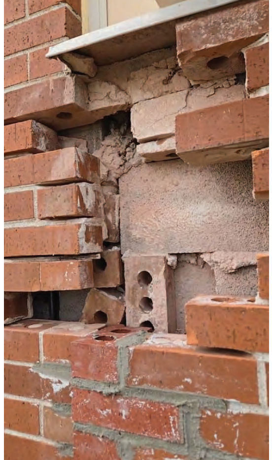
6. New brick at window bump-out with extra brick filling in CMU gaps.
