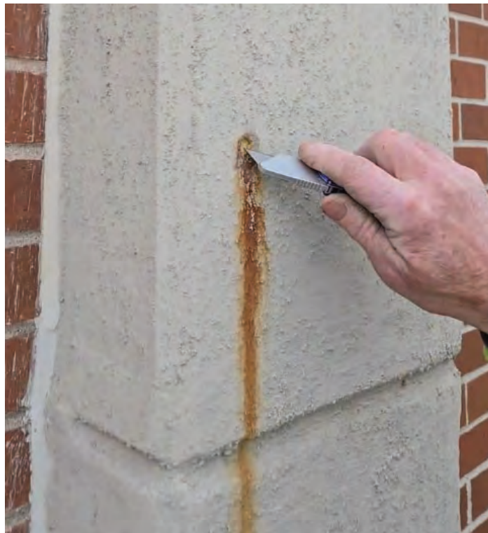
12. Rusting hole in concrete column.
