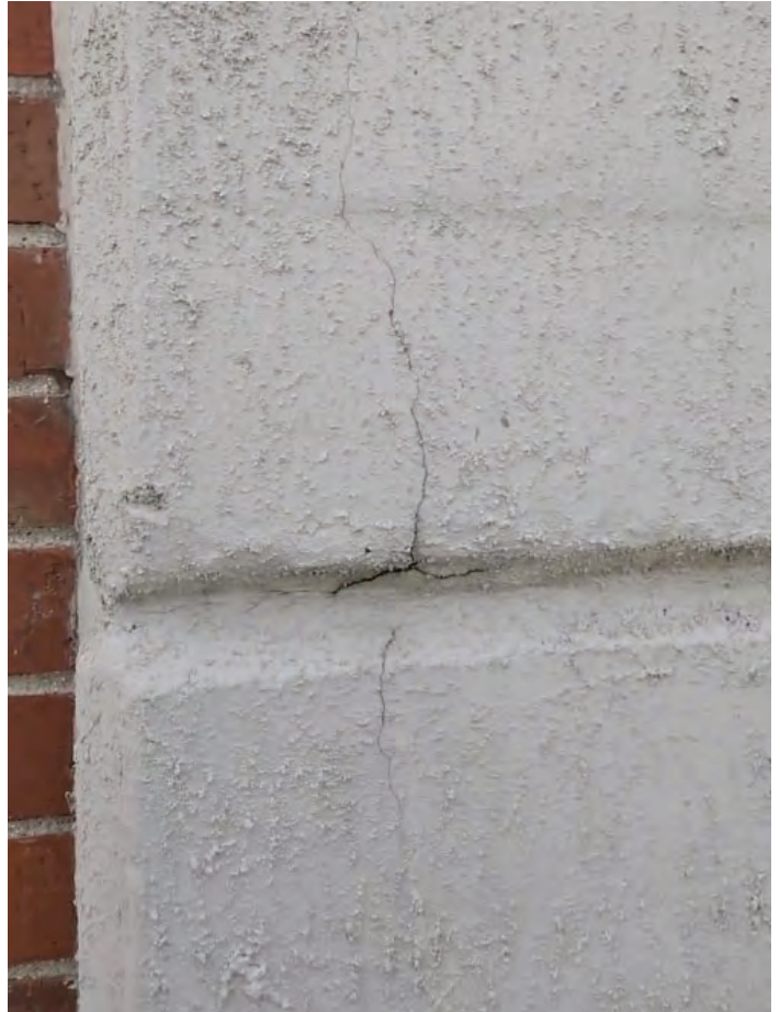
4. Column spider web cracks are stable.
