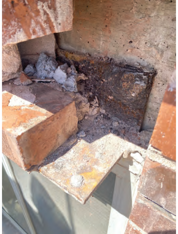
4. 11-story south wall exposed lintel right of Column 11-13 at 9th floor window.
