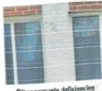
Other concrete deficiencies (e.g., deterioration at edges of beams or columns, spalling, rust spots due to holes or cracks)
