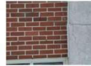
Damaged mortar joints
