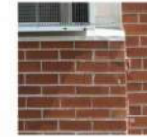
Vertical cracking in masonry, above or below windows
