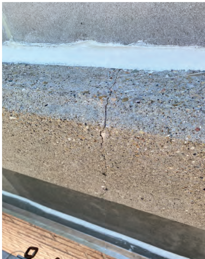
14. Minor concrete crack requiring protective layer (typical).
