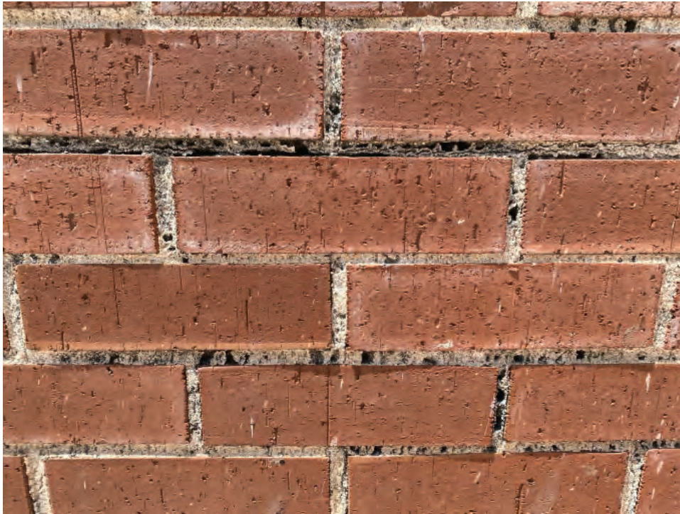
9. 1-story southeast elevation deteriorated mortar.
