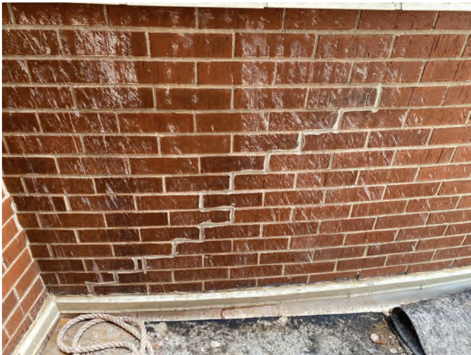
10. 1-story southeast elevation sealant over mortar.
