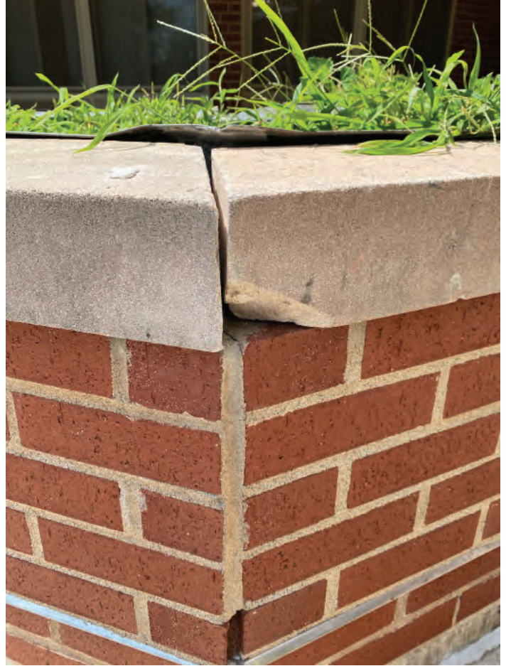
12. Planter stone top with broken corner.
