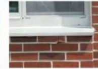
Damaged mortar joints
