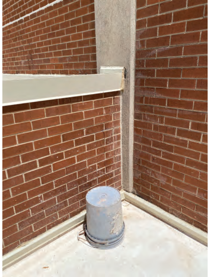
8. 1-story southeast elevation cracked brick.
