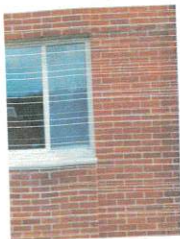
Vertical cracking in masonry above or below windows
