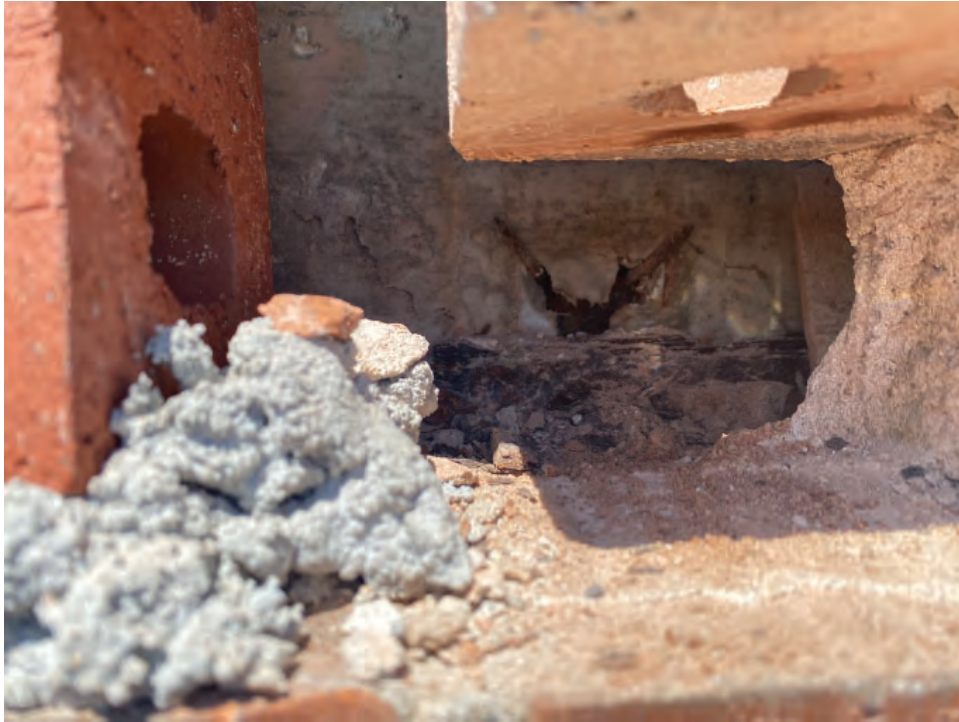
5. 11-story south wall delaminating lintel left of Column 11-13 at 10th floor window.
