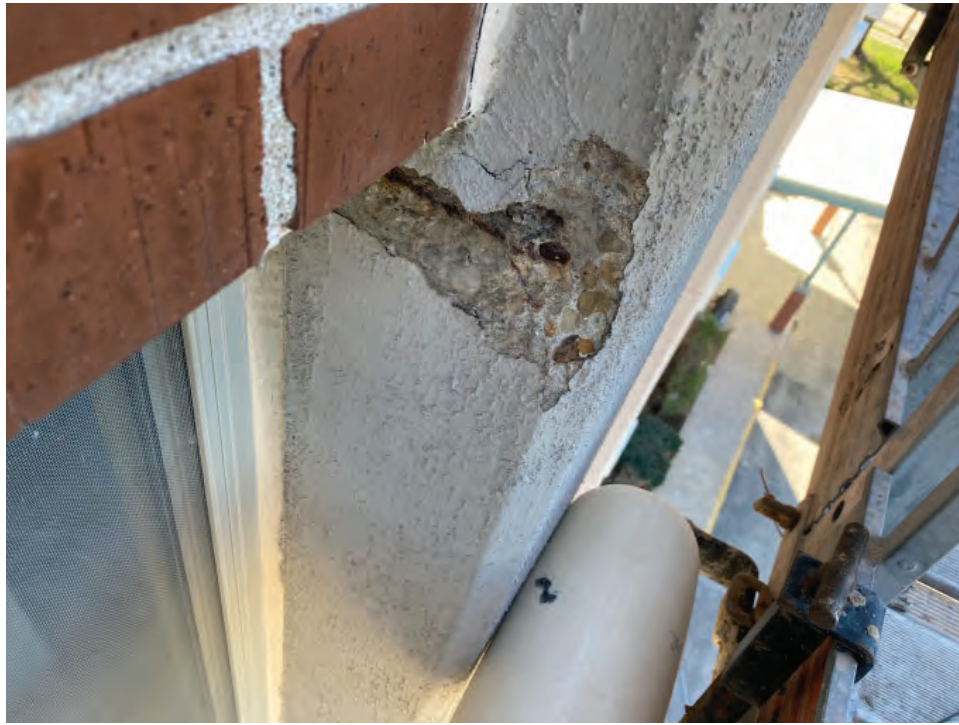
11. 11-story north wall significantly cracked concrete uncovered left of Column 11-8 above 5th floor window.
