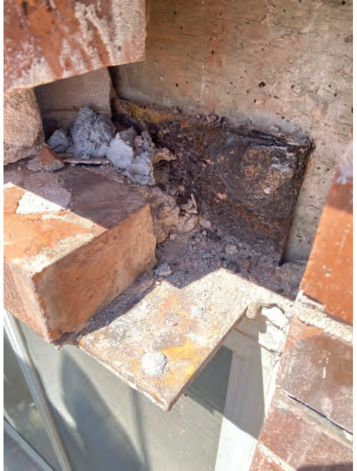
4. 11-story south wall exposed lintel right of Column 11-13 at 9th floor window.
