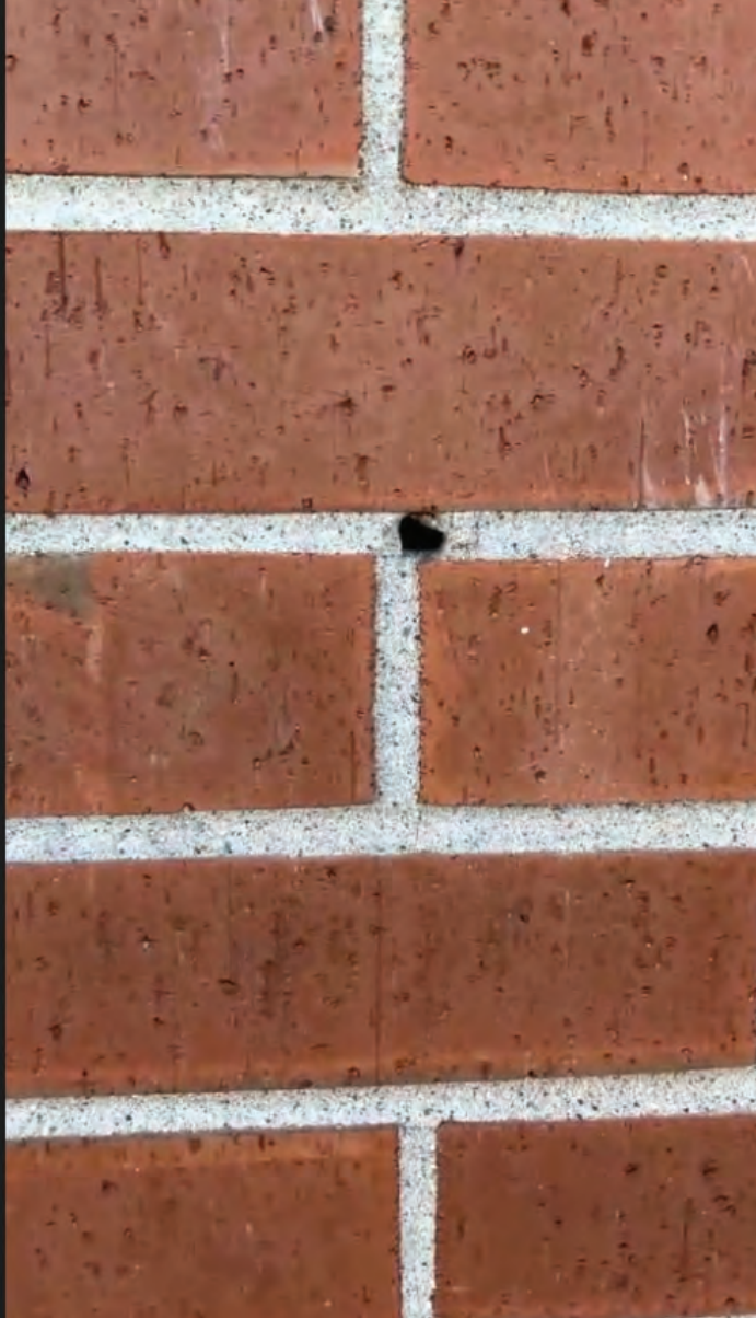
7. Weep hole without visible wick (typical).
