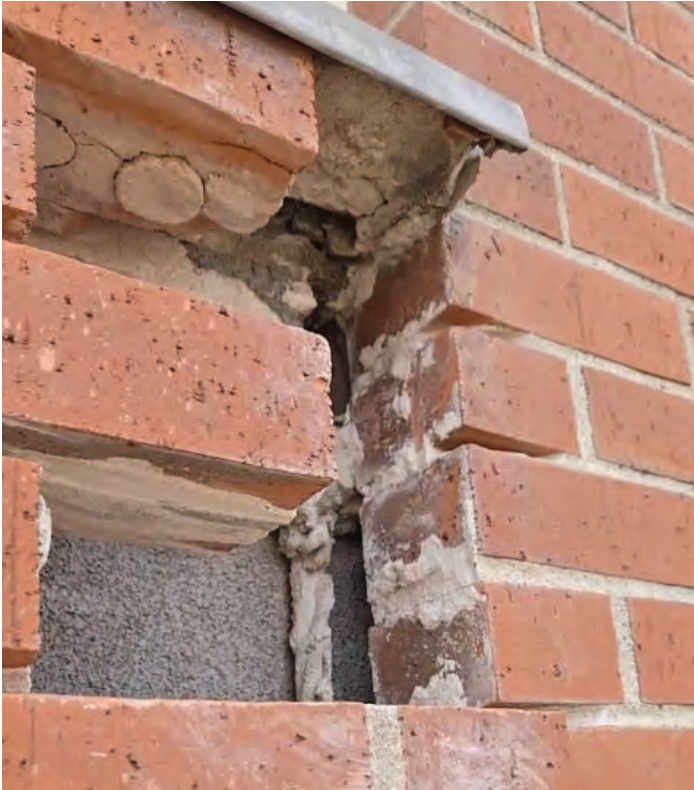
7. Extra layer of brick does not extend beyond the bump-out.
