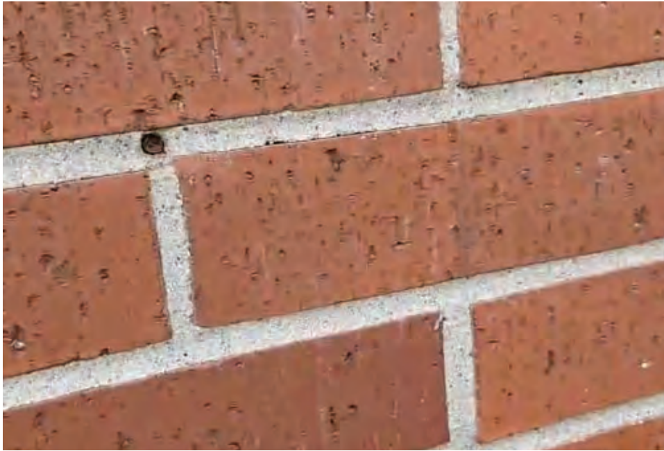
11. Weep holes open but contain debris.
