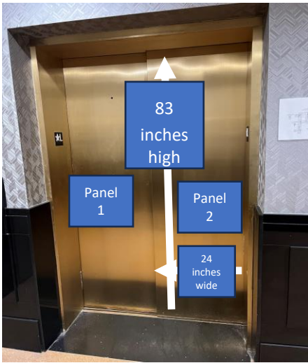
Outside Elevator Door From Lobby Dimensions 2 panels Both 83 inches high X 24 Inches wide
