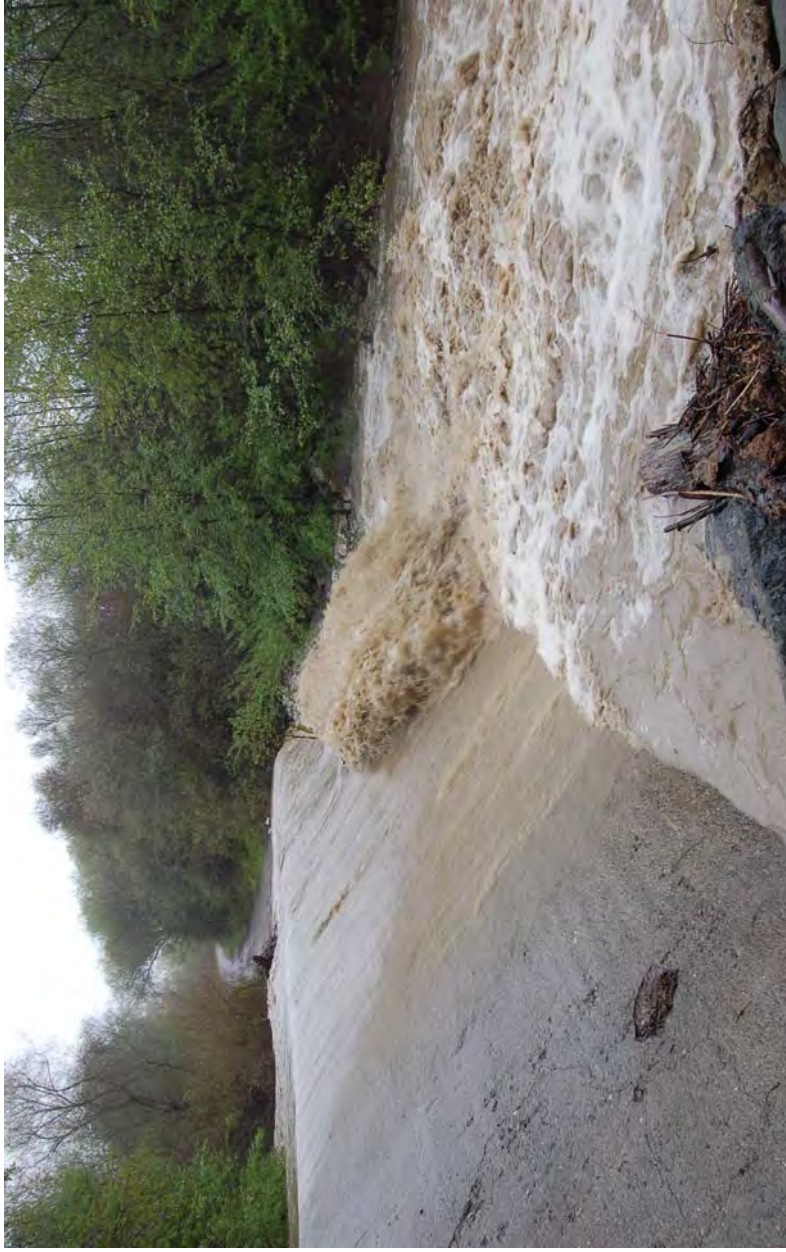
Figure 16. Ferrasci Road crossing during high flows in the spring of 2005.
