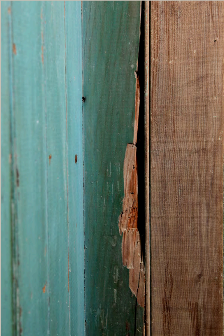
Damaged wooden plank by the NW corner
