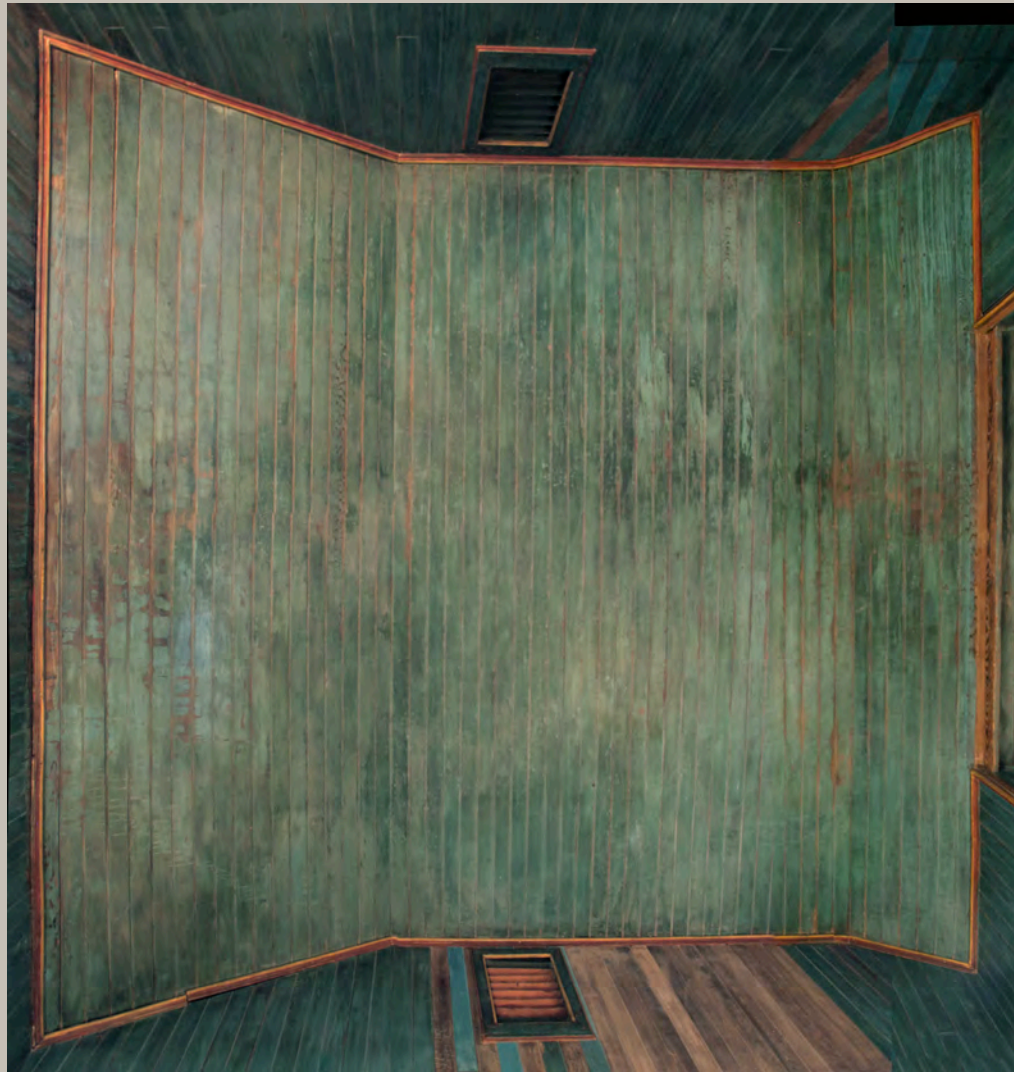
Composite photograph of the ceiling before restoration
