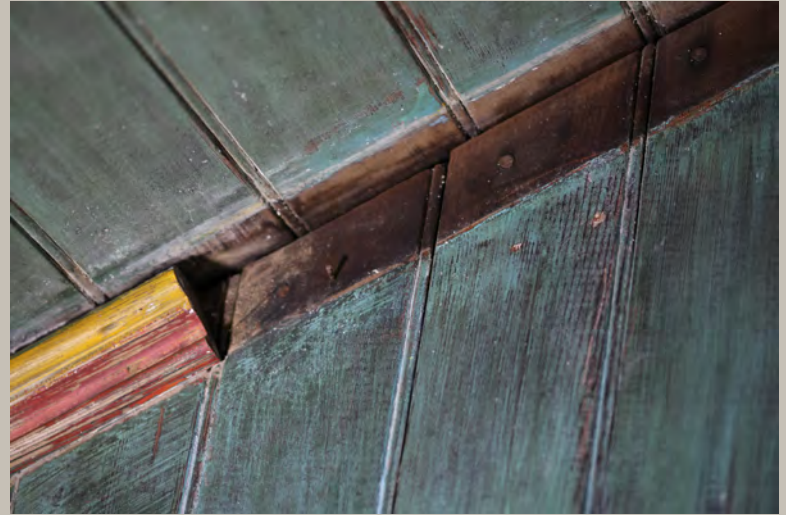
Unpainted wood beneath a temporarily removed section of molding on upper left side of the south wall
