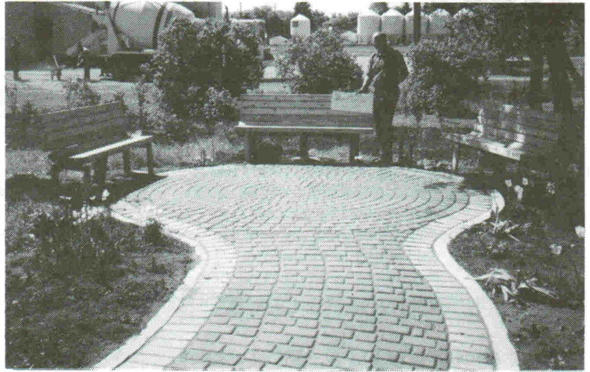
Heritage Park in progress. The cement had dried, the extra legs removed, the park is now ready for sitting!!
