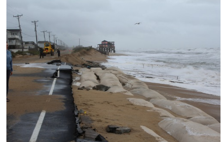
Erosion mitigation on NC 12 in Kitty Hawk, NC, Oct. 2015. Photo: County of Dare.
