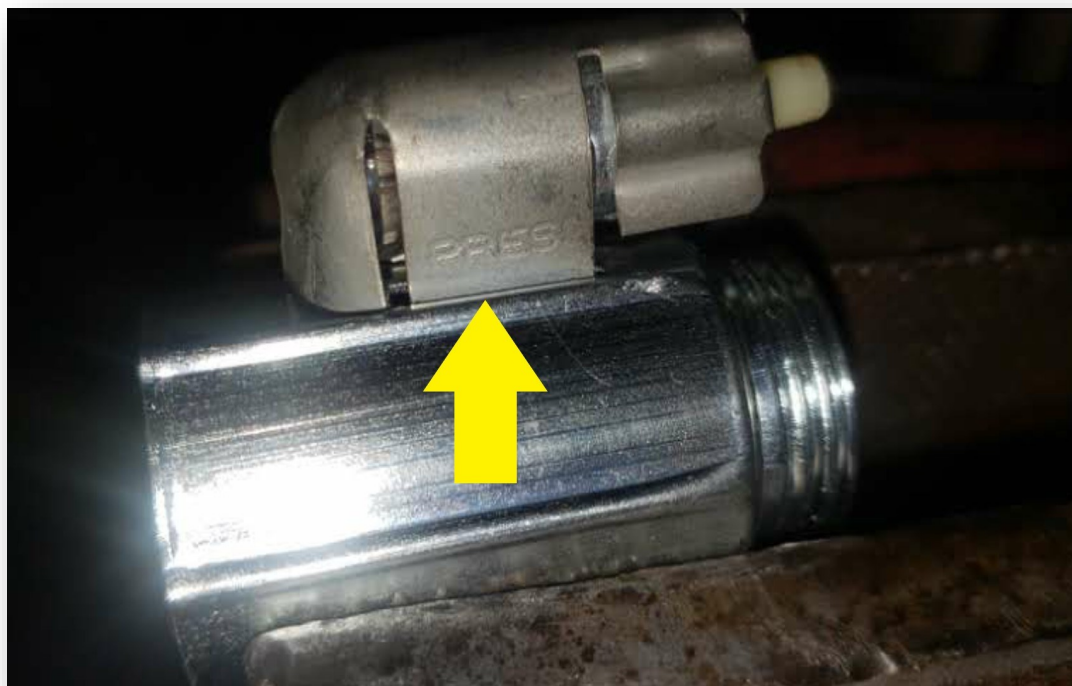
This is where I added solder so that the bulb housing would make good electrical connection. You can see the holder is stamped "PRESS". You pinch both sides and it compresses so it can be removed from the lower housing. After replacing the bulb, the holder would not spring back strong enough to maintain good connection to ground
