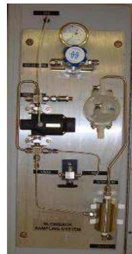
(Blow Back Sample System)
