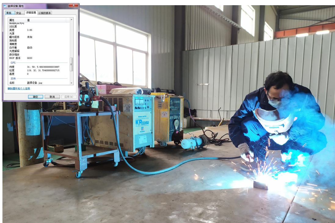
Argon arc welding equipment 4 sets
