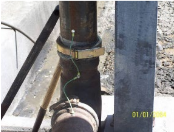
Flexible Elbow (with bonding wire) (Source: OSHA HRT)
