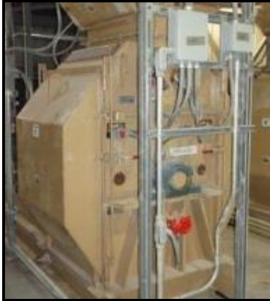
Hammer Mill (Source: OTI)
