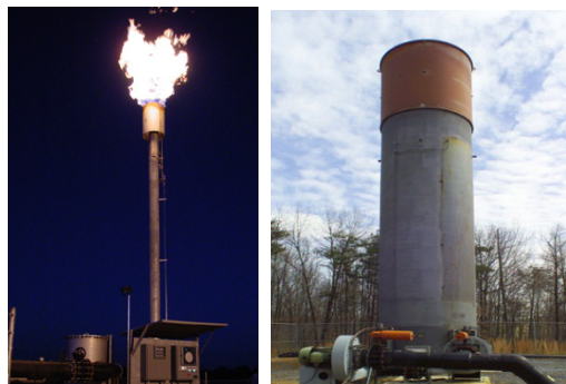
Figure 1-4. Open (left) and Enclosed (right) Flares
