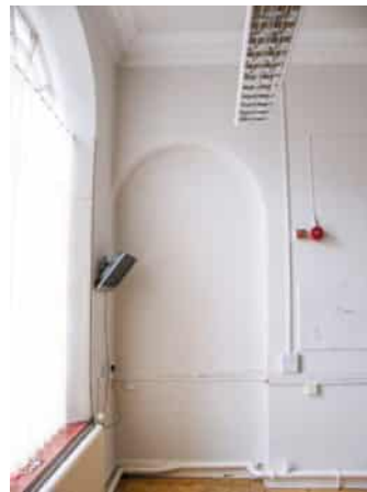
Photo 16: Blocked opening to east of G1
