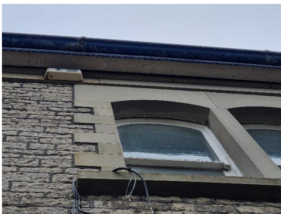
Figure 7 – Gap between fascia and wall (Target Note 2).
