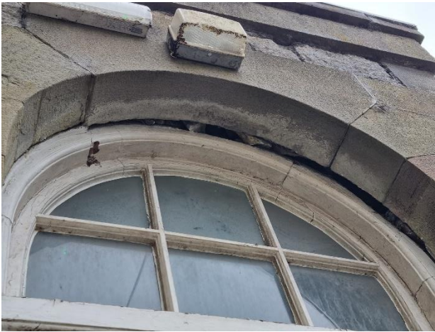
Figure 10 - Gap above window (Target Note 1).
