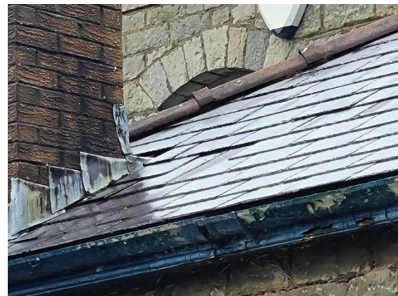
Figure 8 – Gaps around chimney (Target Note 3).
