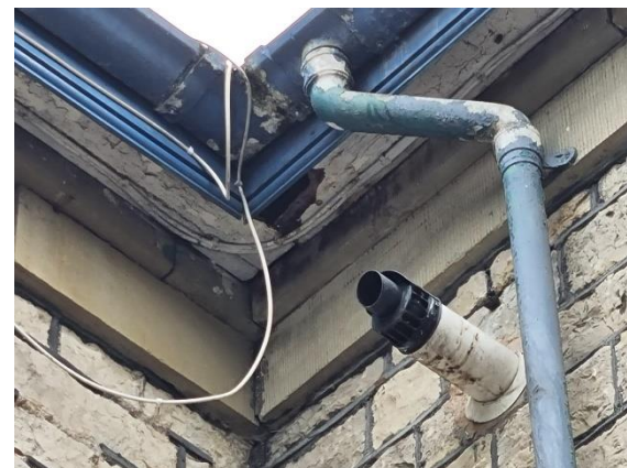
Figure 6 – Hole in soffit on Building A (Target Note 6).
