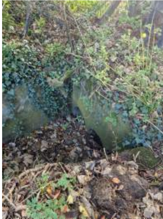
Debris within the existing twin culvert outfall – taken 27/10/2025
