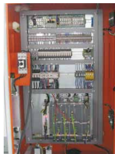
CE-Marked Electric Cabinet
