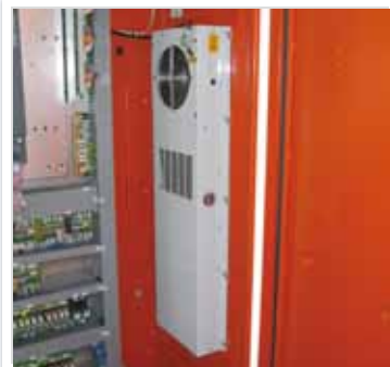
Built-In Heat Exchanger
