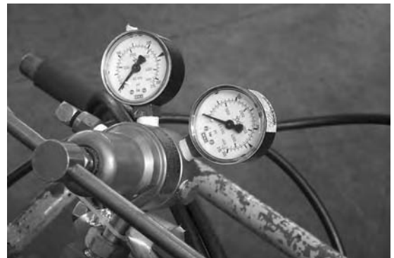
Figure 1.23 Pressure gauges graduated in bar and in psi.
