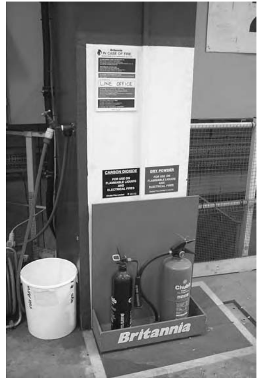
Figure 1.18 Typical aircraft hangar fire point.
