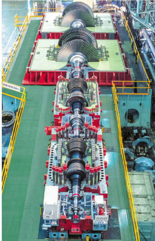
Figure 1.3 700 MW ST Hekinan Unit 3, Chubu Electric Power Co. Source: Reproduced by permission of Mitsubishi Hitachi Power Systems America, Inc.
