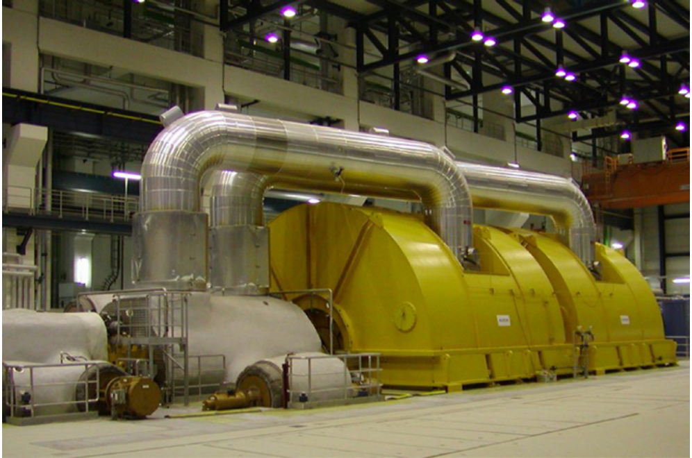
Figure 1.1 Alstom steam turbine. Source: Reproduced by permission of Alstom.
