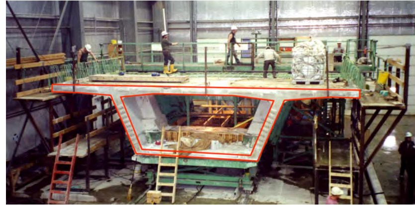
Figure 54.11: Deviation segment in the precasting facility. The basic cross-section has been highlighted.
