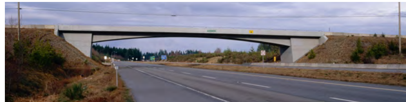
Figure 7.3: Royston Road Underpass, B.C. (A photograph of the bridge depicted in the drawing of Figure 7.2).
