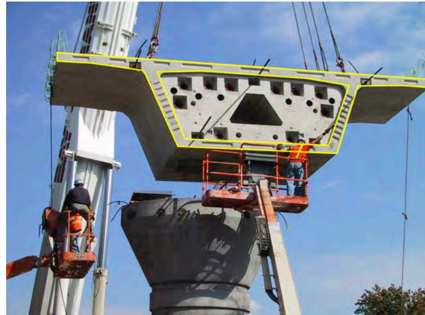
Figure 54.10: Pier segment being erected onto a pier. The basic cross-section has been highlighted.
