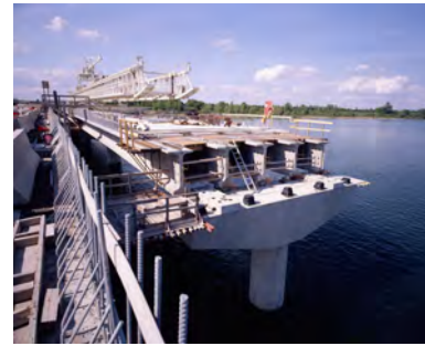
Figure A.6: Application of precast concrete I-girders (with cross-section similar to the one shown in Figure A.5) in bridge construction
