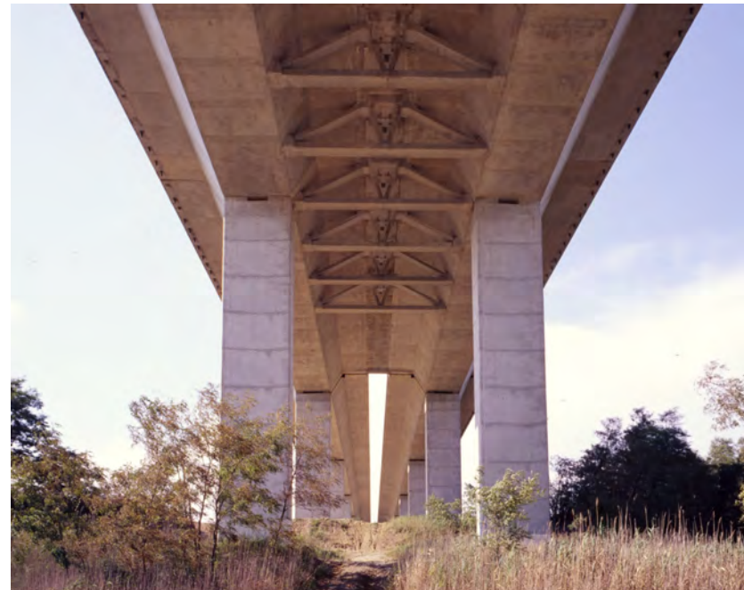
Figure 48.2: Bridge piers constructed from precast box pier segments. Note the horizontal joints between the segments. Chesapeake and Delaware Bridge, USA.
