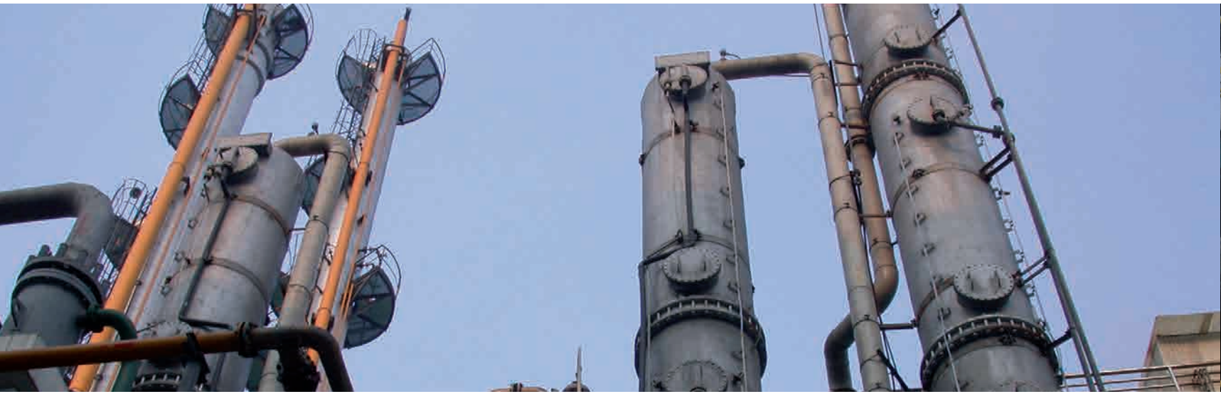
Expansion of the Olefin Cracker for Repsol YPF Tarragona (Spain).
