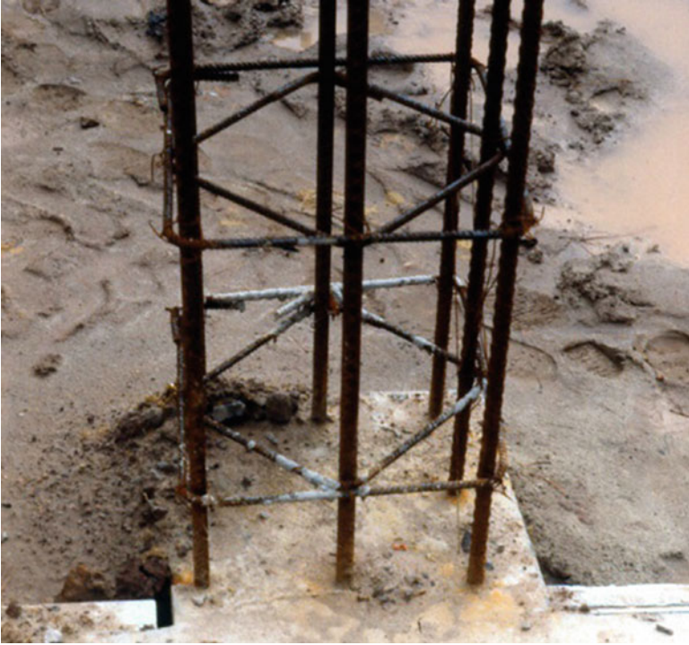
Figure B5.2 Main reinforcements and Ties for a column with 8 bars (see Figure 5.12e)
