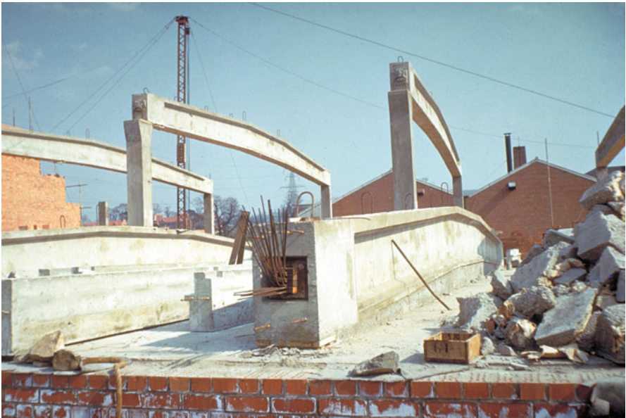
Figure B9.3 Post-tensioned concrete beams Courtesy of the William G. Godden Collection, NISEE-PEER, University of California, Berkeley
