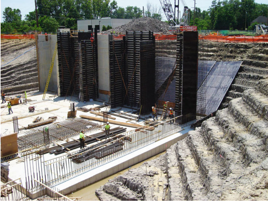
Figure B8.1 Large wall forming Courtesy of Mr. Doug Peters PE, President, Christman Constructors, Inc.
