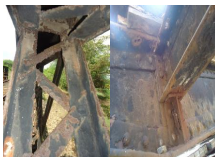
Figure 1: Corrosion on the bridge members
