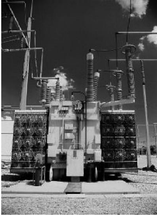
FIGURE 4.16 A large power transformer. Source: http://images.google.com/images?q=photos+of+power+transformers
