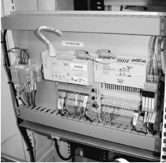
FIGURE 8.2 Example PLC installation.
