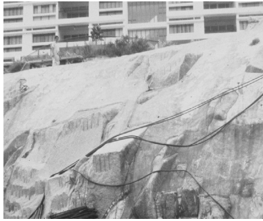
Figure 6.3 'Chunam' rock face protection (Hong Kong).
