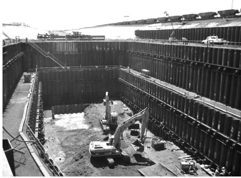
Figure 6.19 Deep anchored sheet-pile excavation, Port Headland Western Australia. (Image courtesy of Marc Woodward, Perth.)
