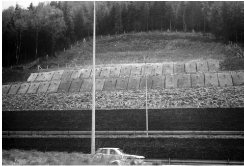
Figure 6.37 Precast slabs used with anchors to provide a retaining structure at the toe of a failing slope (South Wales).
