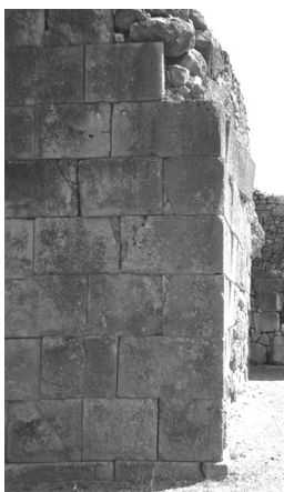
Figure 9.6 Start of toppling failure in an ancient masonry block wall in Delphi, Greece.
