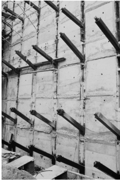
Figure 6.27 Top-down construction using anchored steel H piles in-filled with cast in situ concrete planking (Hong Kong).
