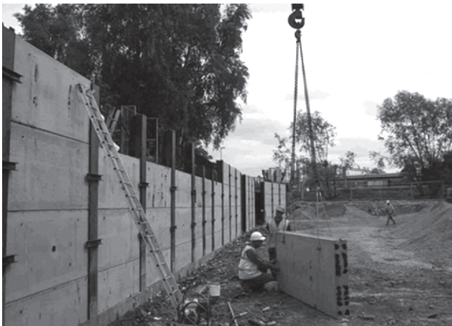
Figure 6.26 King post wall. (a) Plan showing steel H-piles and concrete panels. (b) Wall construction, using pre-cast panels. (Image courtesy of ElecoPrecast.)
