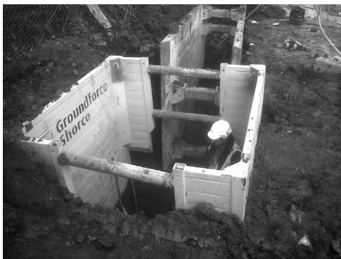
Figure 6.13 Trench support provided by manhole and trench shields (image courtesy of VP plc).
