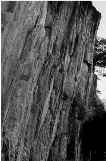
Figure 6.2 Overhanging, unsupported rock face in school playground (Hong Kong 1981).
