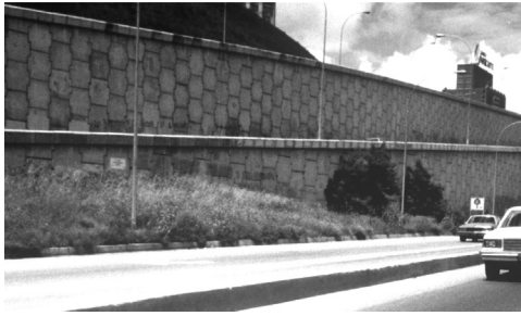
Figure 6.32 Reinforced earth walls (Caracas, Venezuela).
