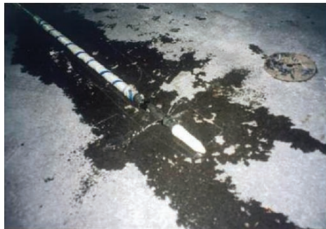
Fig. 15.24. Example of nozzle for injection of liquid (at site of Penta-Ocean Inc.)
