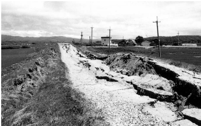
Fig. 13.5. Damage to a river dike at the Shiribeshi-toshibetsu river, Hokkaido, Japan, during Hokkaido-Nansei-oki earthquake of 1993
