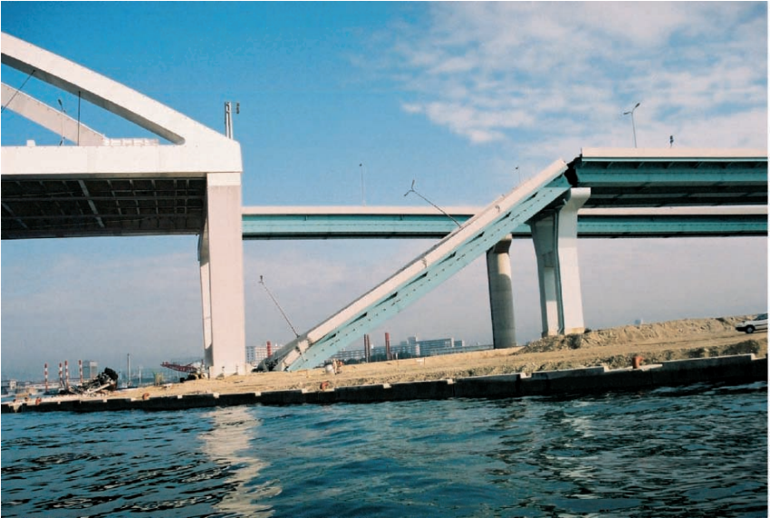
Fig. 13.16. Damage to an access to a bridge at Kobe-Nishinomiya during 1995 Hyogoken-Nambu earthquake
