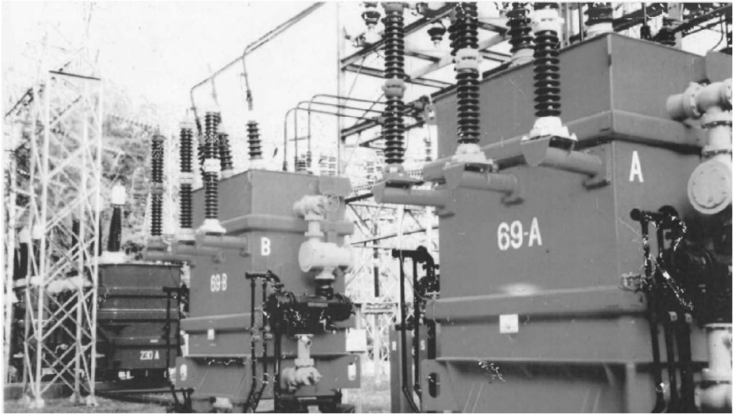
FIGURE 1.15 Substation power transformers.
