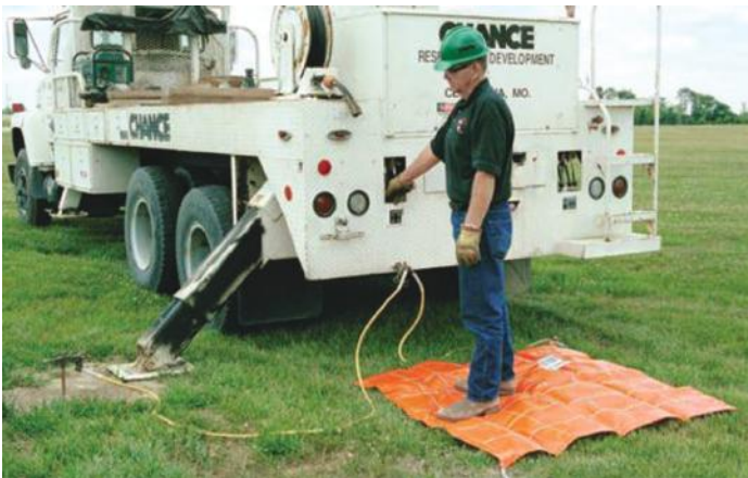
FIGURE 8.21 Worker standing on ground mat attached to truck. (Chance® tools and grounding equipment depicted courtesy of Hubbell Power Systems, Inc.)
