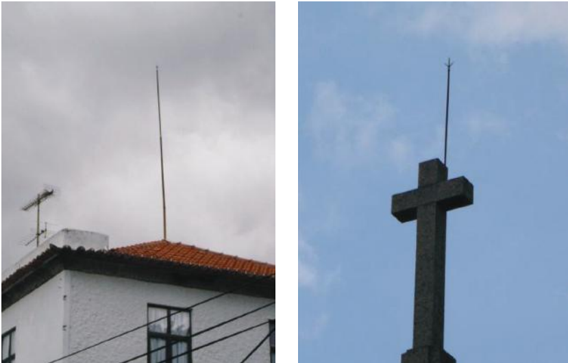
FIGURE 11.5 Lightning pole on top of buildings.
