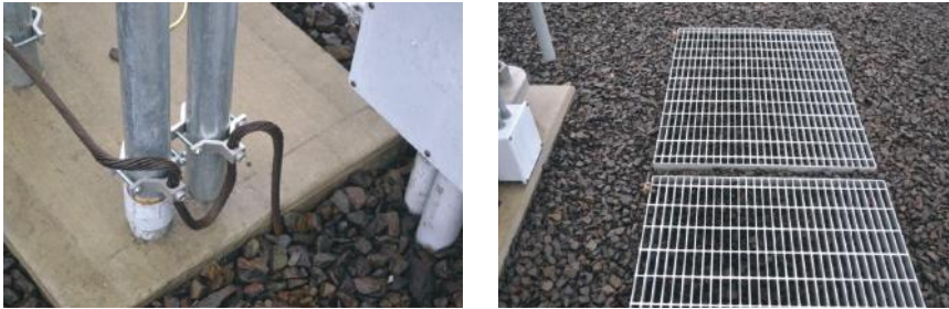
FIGURE 12.88 (a) Bonding gate to ground grid and (b) grounded standing platform.
