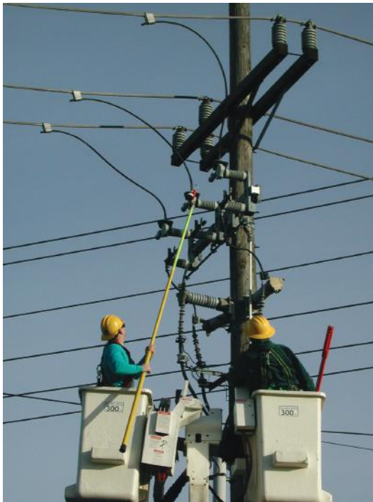
FIGURE 9.5 Using hot stick in insulated aerial baskets. (Courtesy of Seattle City Light.)
