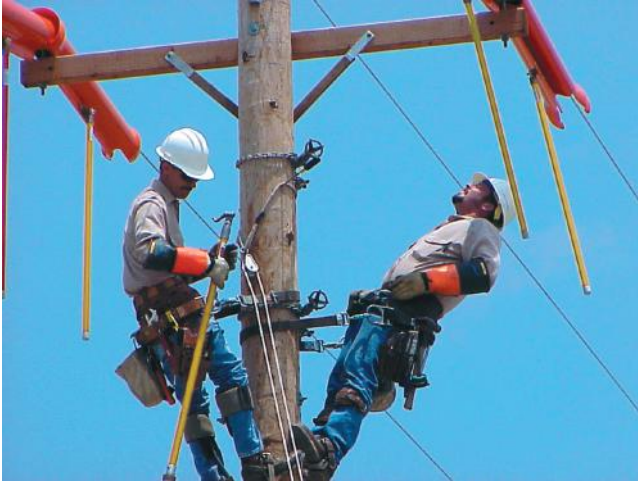
FIGURE 9.8 Workers with PPE and IPE. (Courtesy of Salisbury by Honeywell, Bolingbrook, IL.)
