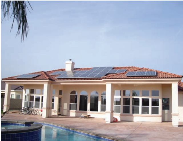
FIGURE 33-3 Rooftop array of modules. (Delmar/Cengage Learning)
