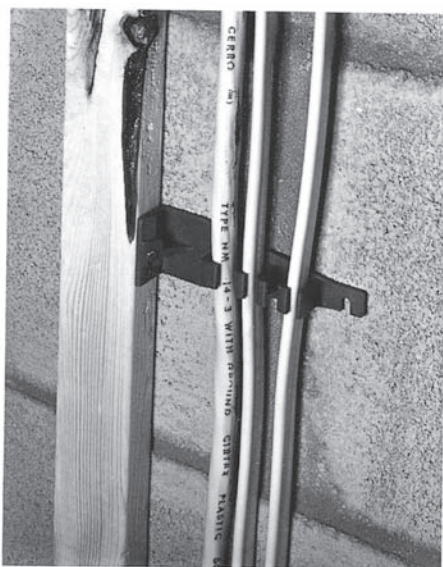
FIGURE 4-27 Devices that can be used to meet the Code requirement to maintain a 1¼-in. (32-mm) clearance from framing members. (Delmar/Cengage Learning)
