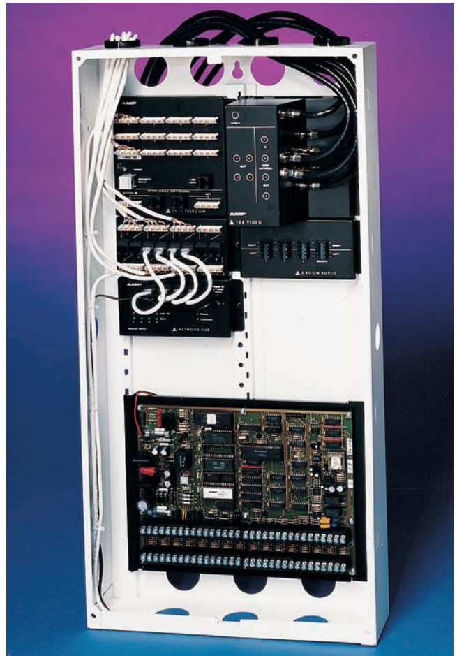
FIGURE 31-6 A “service-center” is the hub of a structured wiring system with telecommunications, audio, video, and home automation controllers installed. (Courtesy Leviton)
