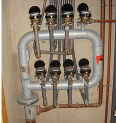
This new manifold for water meters has replaced the old one after 4 years of use, having been connected directly to a copper pipe in the building (0.85 V of potential difference, see the point of corrosion in the bottom left). With a PVC battery support, lifetime is unlimited.
