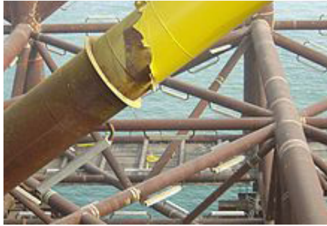
Sacrificial anodes mounted “on the fly” for corrosion protection of a metal structure
