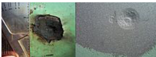
A corrosion pit on the outside wall of a pipeline at a coating defect before and after abrasive blasting.
