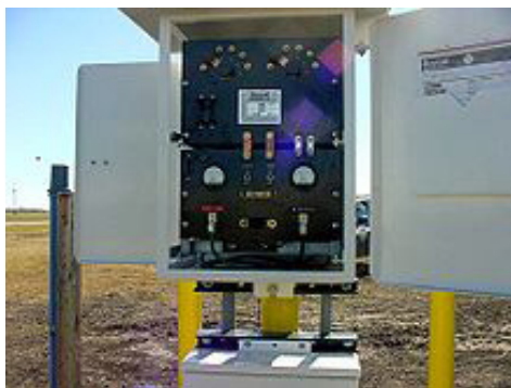
Electrical panel for a cathodic protection system
