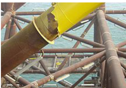
Aluminum anodes mounted on a steel-jacketed structure
