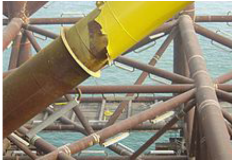
Aluminium sacrificial anodes ( light colored rectangular bars ) mounted on a steel jacket structure.
