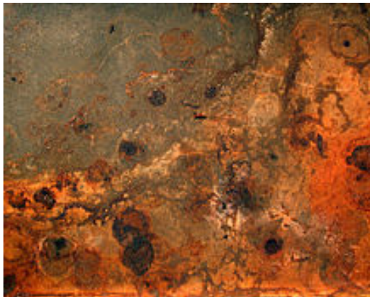
Rust, the most familiar example of corrosion.
