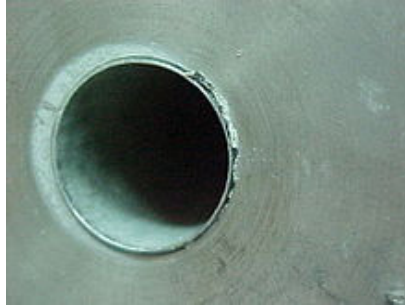
Corrosion in the crevice between the tube and tube sheet (both made of type 316 stainless steel) of a heat exchanger in a seawater desalination plant.
