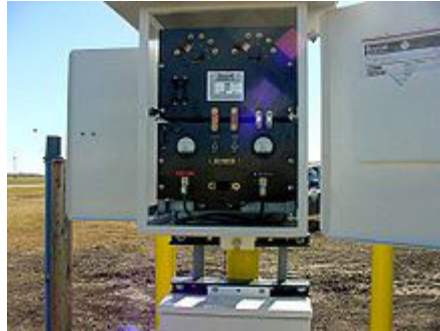
An air cooled cathodic protection rectifier connected to a pipeline.
