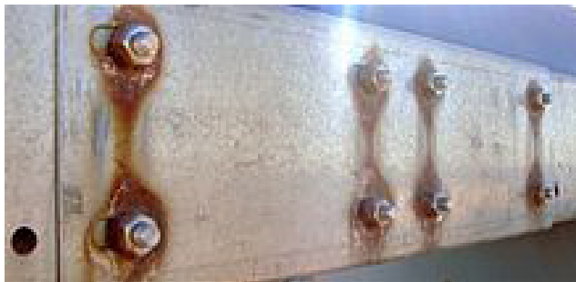
Stainless steel cable ladder with mild steel bolts
