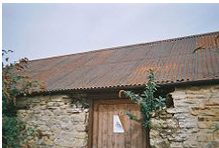
Rusted corrugated steel roof
