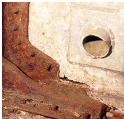
Galvanic corrosion of aluminium. A 5-mm-thick aluminium alloy plate is physically (and hence, electrically) connected to a 10-mm-thick mild steel structural support. Galvanic corrosion occurred on the aluminium plate along the joint with the steel. Perforation of aluminium plate occurred within 2 years.
