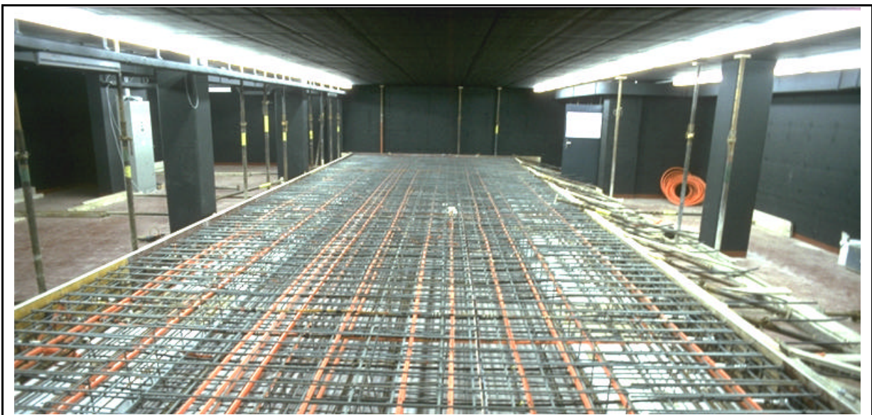
Figure 8.1. The holographic table before concreting. The orange pipes would later contain the optical fibers.
