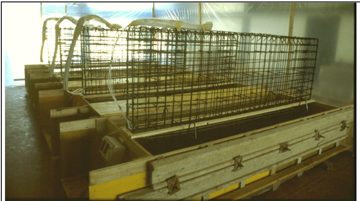
Figure 8.9. Formwork and rebars of the reinforced concrete walls. The white sensor bundles are also visible.
