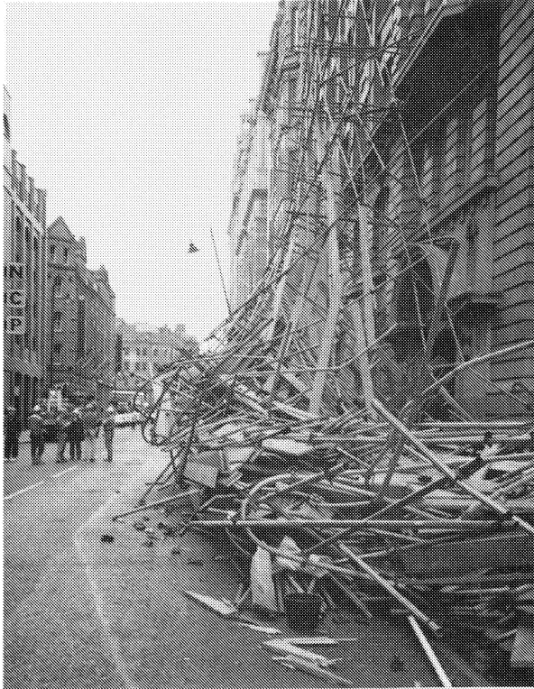
figure 1- the debris was localised
