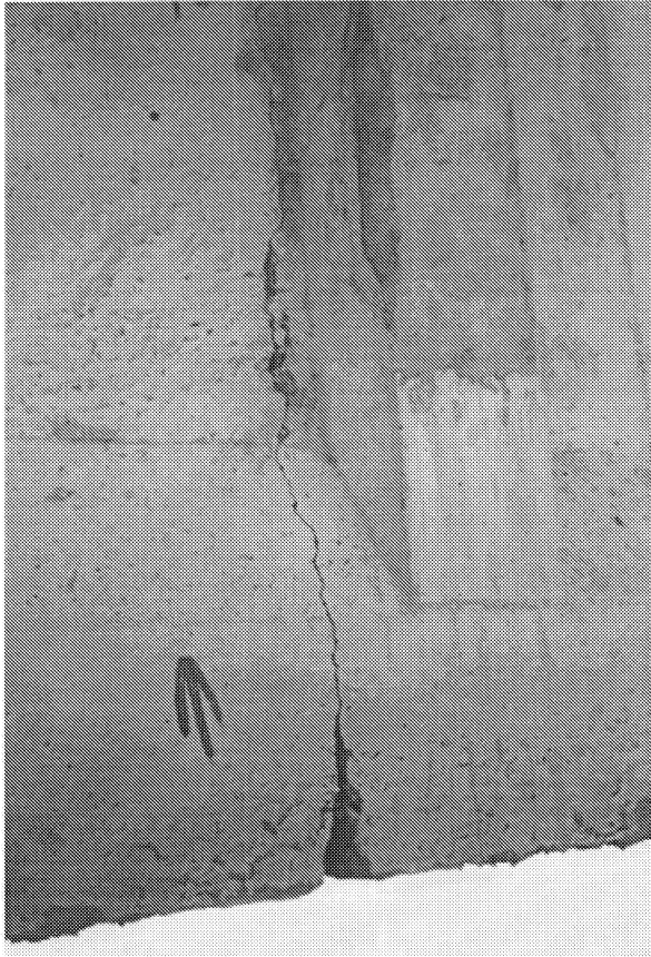
Figure 2. Flexural shear crack in bottom flange and web.
