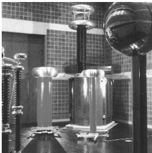
Figure 6.2.1-1: 500 kV/ 125 kVA test transformer with oil-filled tank and with porcelain bushing in the HV test laboratory of Hochschule Würzburg-Schweinfurt.
