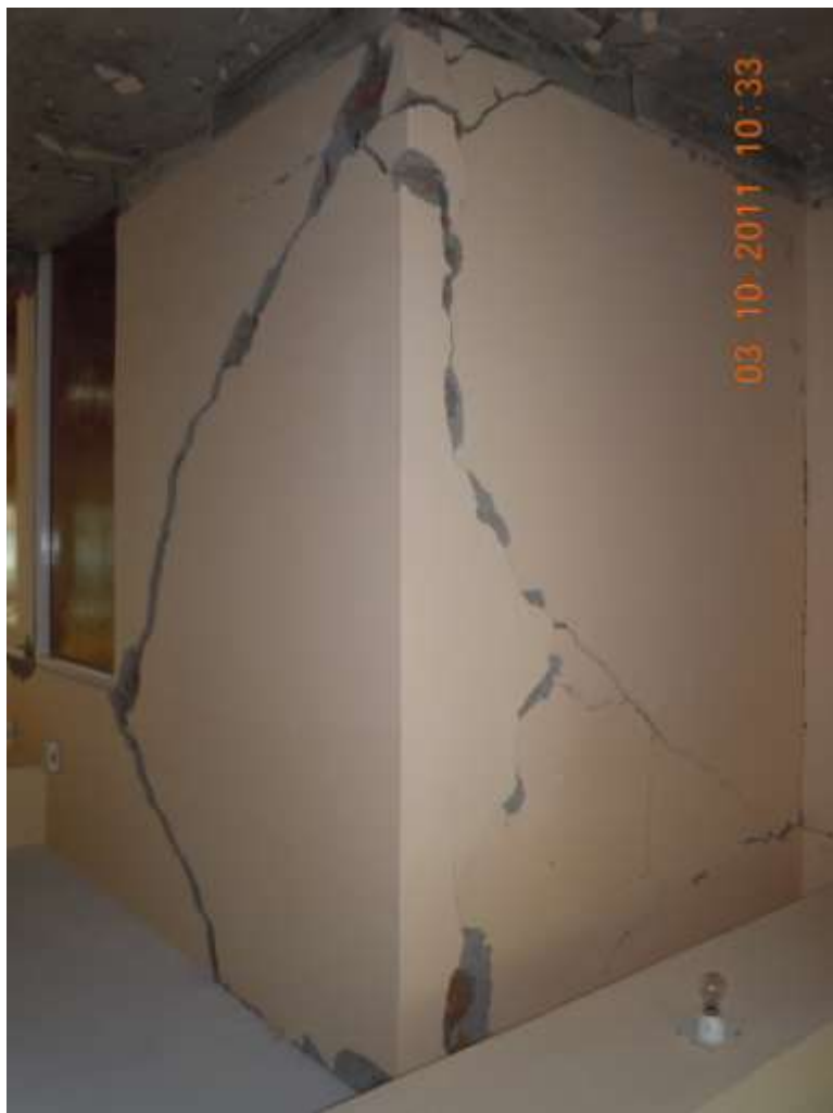
Absence of column at corner
