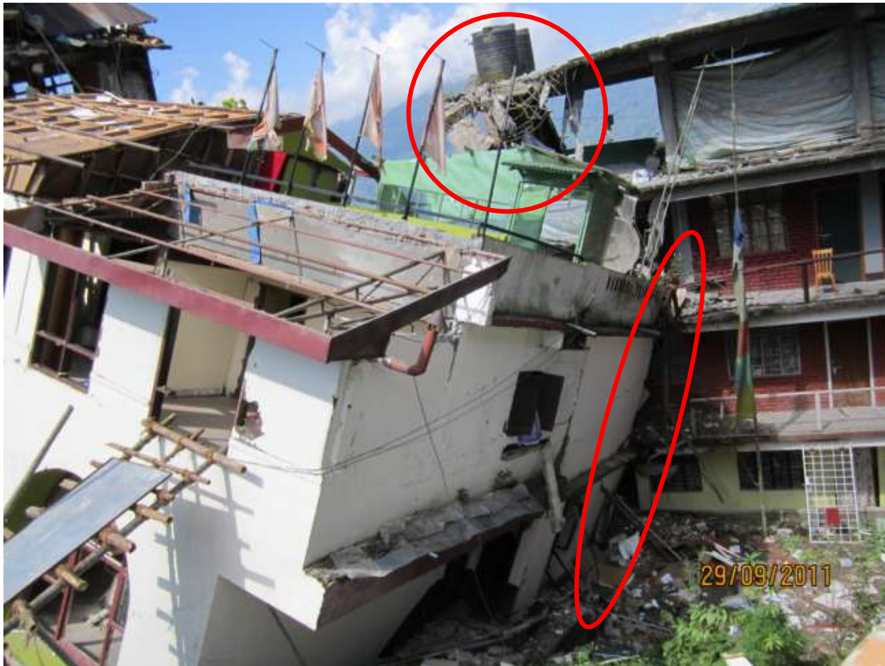
Collapsed building colliding with adjacent one at Balwakhani
