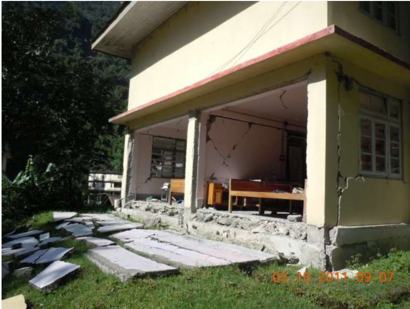
Out-of-Plane Failure of Infill of SDM Quarter at Chungthang
