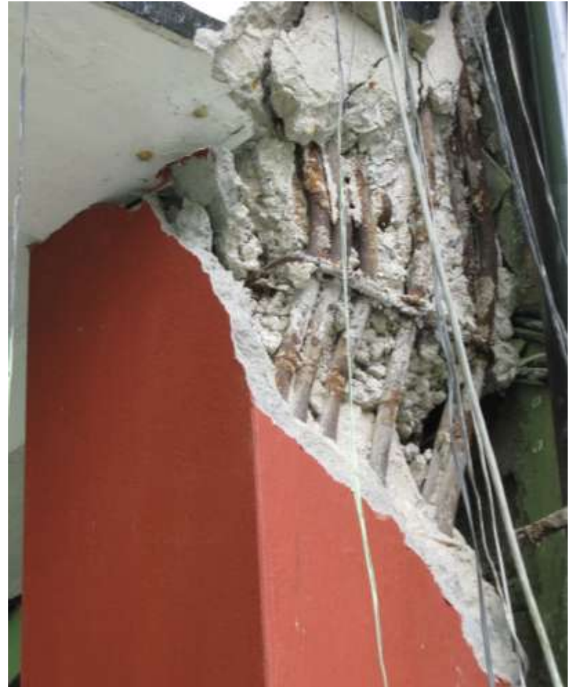
Damage to State secretariat building at Tashiling, Gangtok
