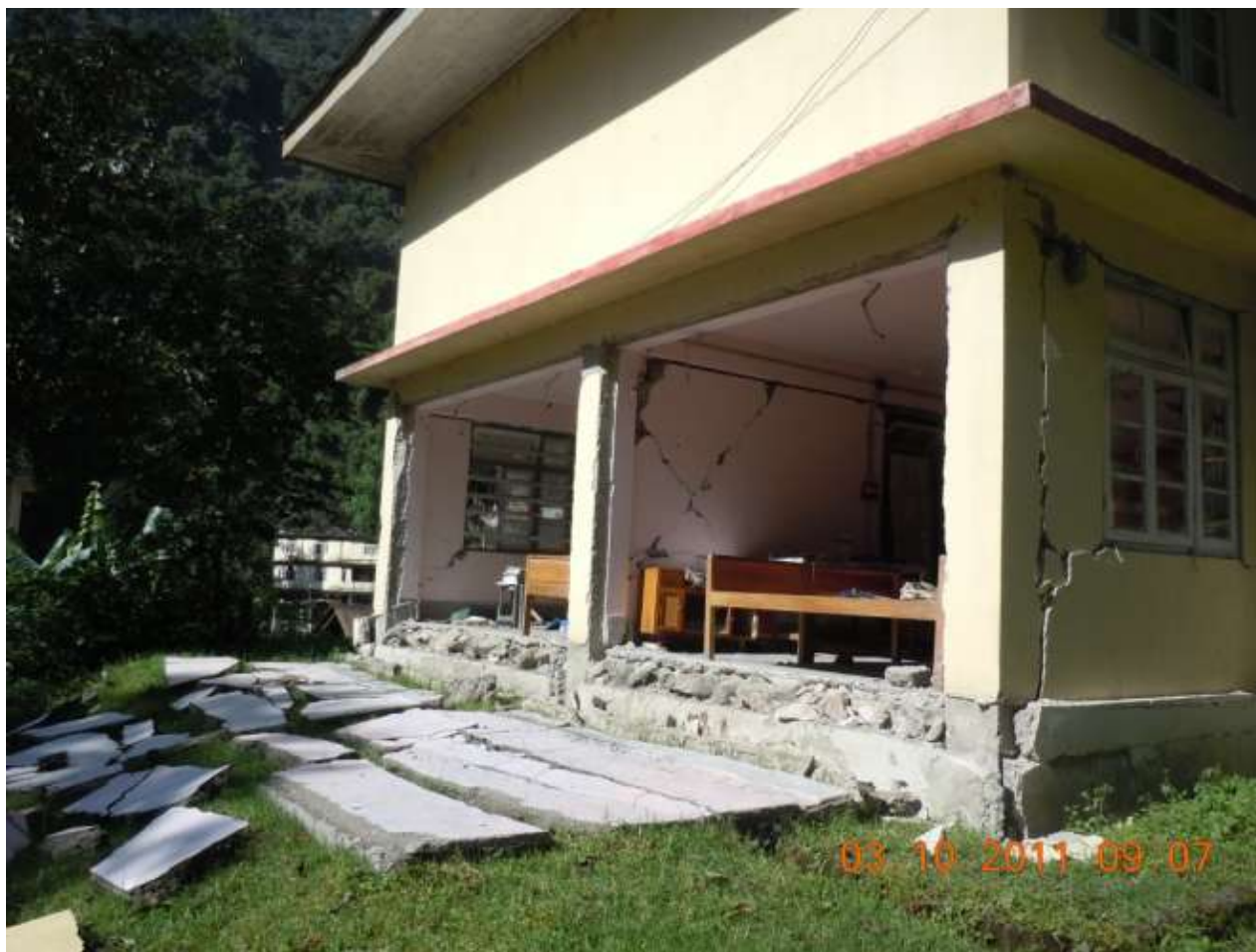
Out-of-plane failure of infill wall
