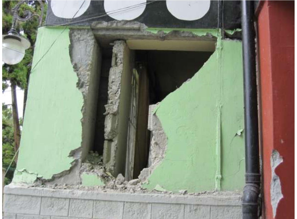
Damage to State secretariat building at Tashiling, Gangtok
