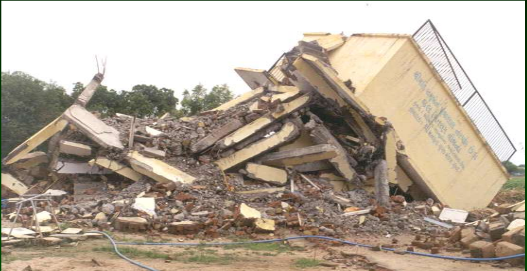
Frame Supported Tank at Manfera
