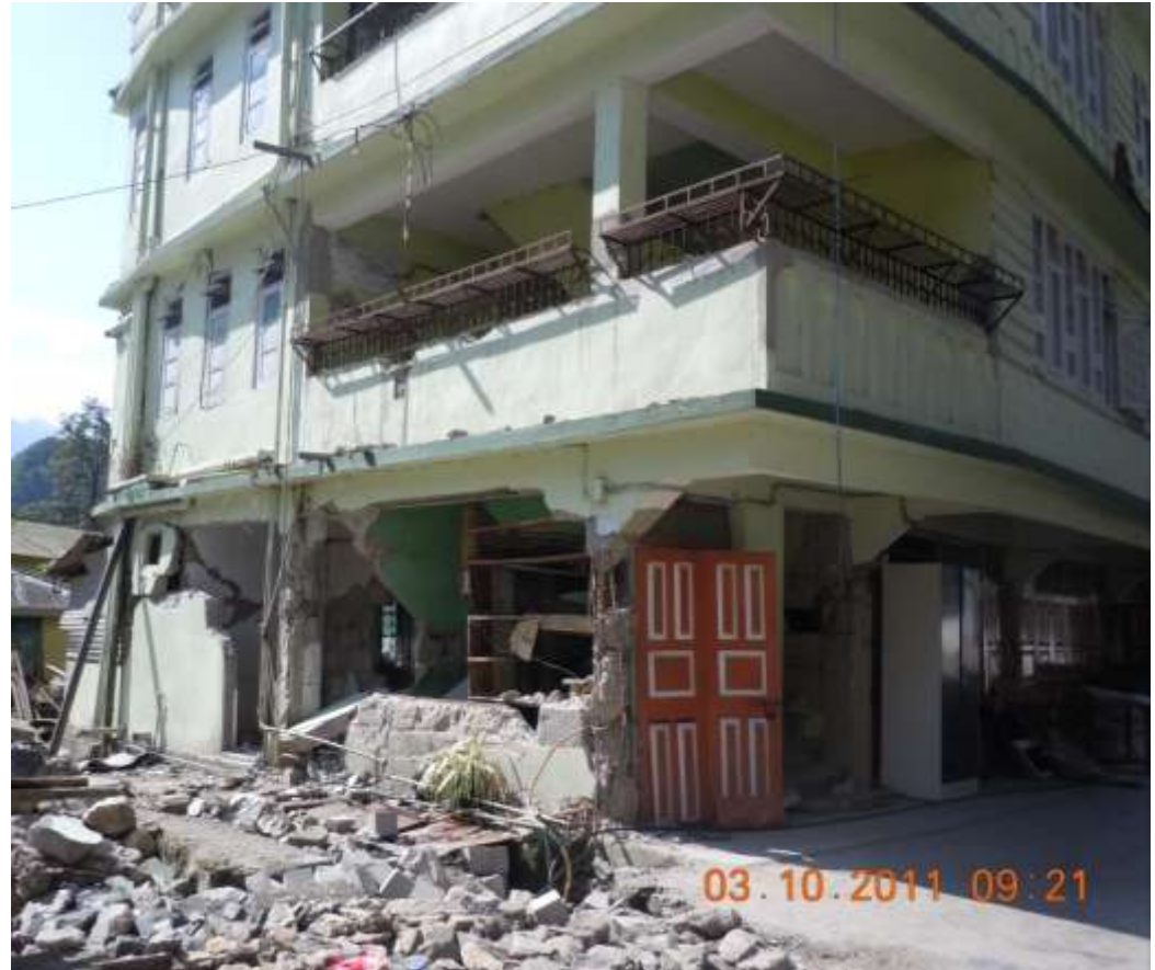
Severe damage in a 5 storey building at Chungthang
