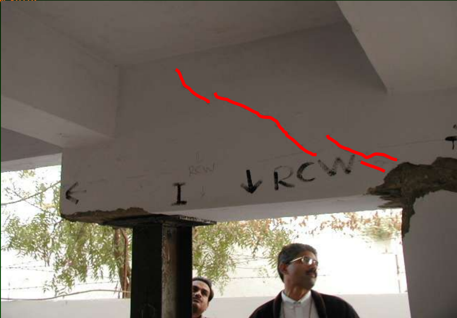
Damage due to Floating Columns
