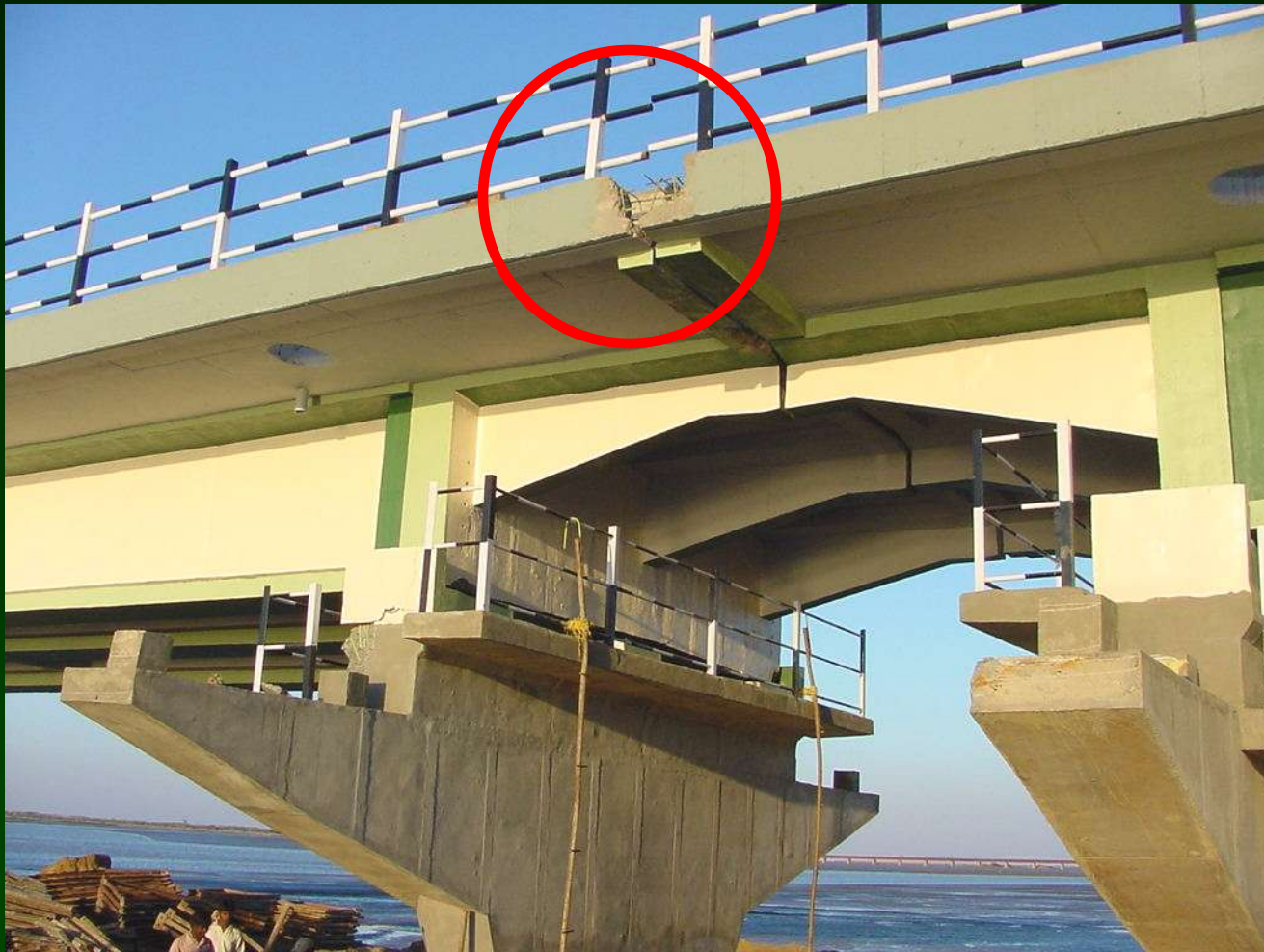
The New Surajbadi Highway Bridge Longitudinal pounding of decks
