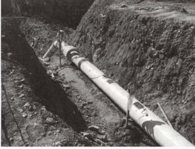
Electrodes used to monitor pipe potential
